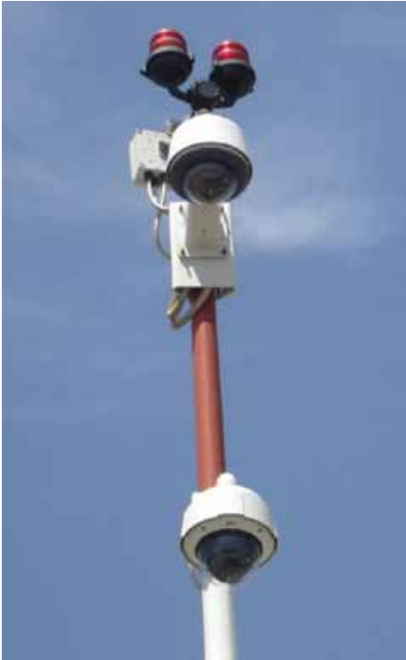
Denver Int'l uses pan, tilt, zoom domes like this unit to enhance terminal security.
