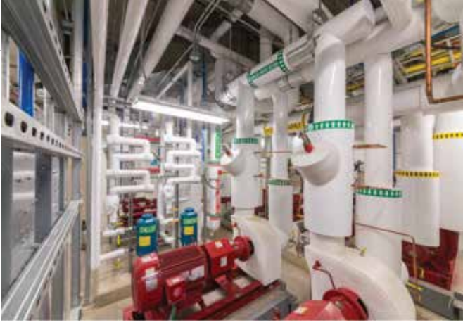
Mechanical systems are grouped in a separate tall section of the base building.
