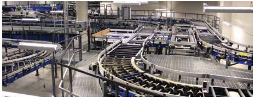
28 Calgary Int'l Looks Forward to Raising Customer Service & Lowering Energy Consumption with New Baggage System
