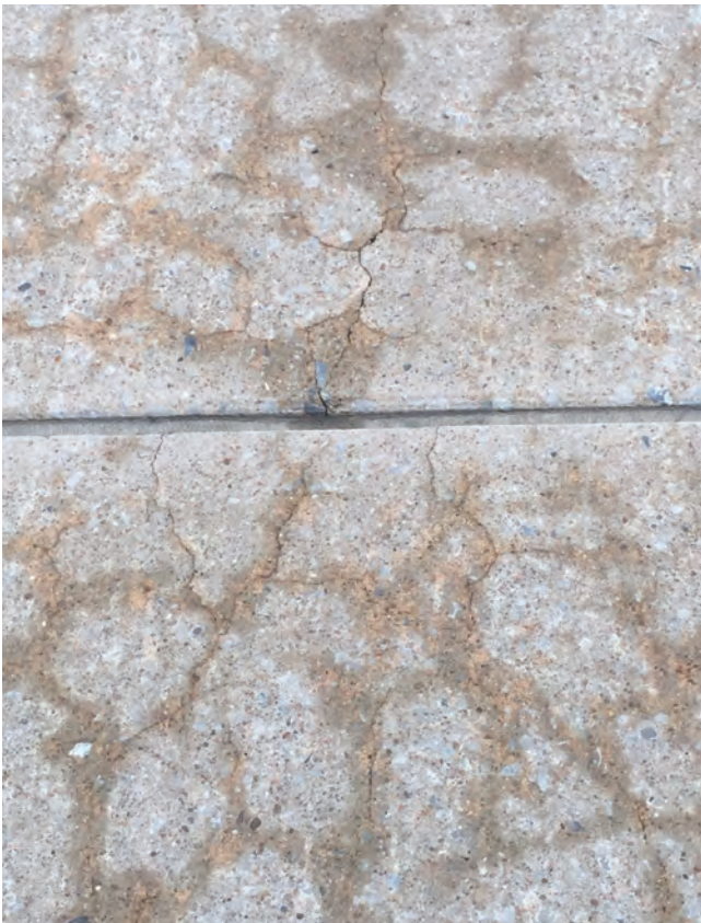
An alkali-silica reaction in the original concrete later caused pronounced damage to the runway and other airfield pavement.
