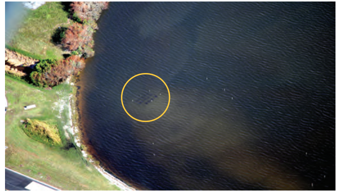
Crews created a new seagrass island with plants harvested from the area that needed to be filled to support the new runway safety area.
