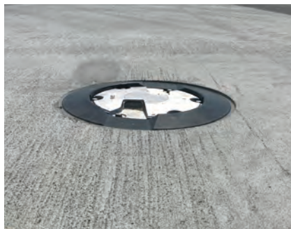
42 Naval Air Station Oceana Converts to LED Airfield Lighting
