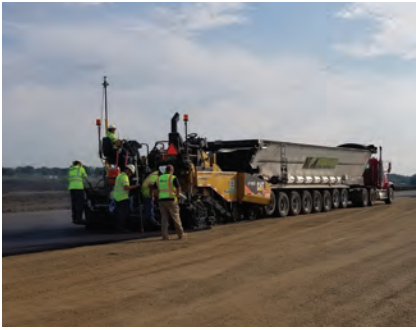
8 New Main Runway at Reynolds Field Improves Safety & Primes Pump for Revenue Growth
