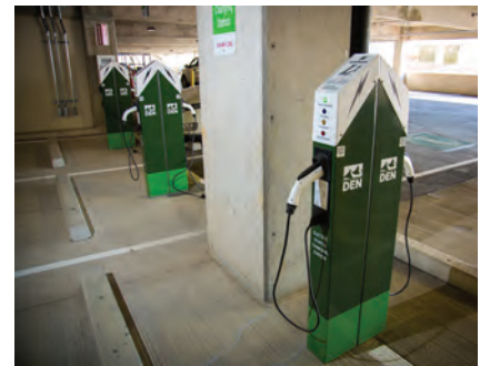
22 Denver Int'l Takes Deep Dive into Power System to Ensure Reliability & Resilience
