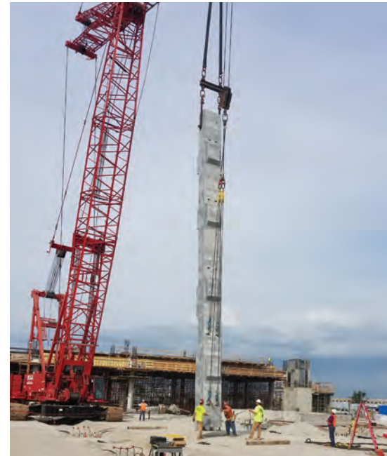
Designers specified high-strength precast concrete columns rather than shear walls to provide horizontal support for the structure.
