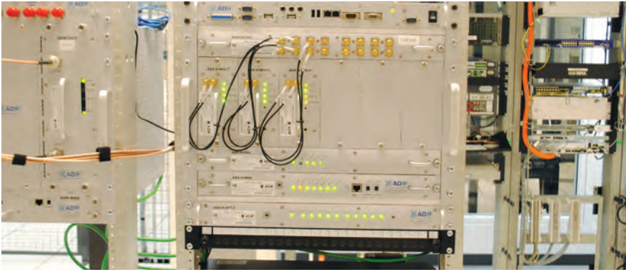
This is the type of DAS system installed at Vancouver Int'l.
