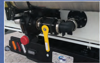
GLYCOL RECOVERY FOR PICKING UP DE-ICING FLUID
