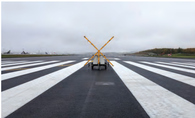
In addition to improving pavement, the airport also installed new runway lighting.
