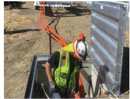
16 San Francisco Int'l Installs New Perimeter Security System
