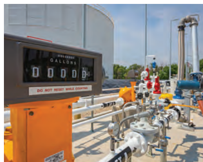
30 Fuel System Upgrades at Mitchell Int'l Benefit Tenant Airlines and Nearby Airports
