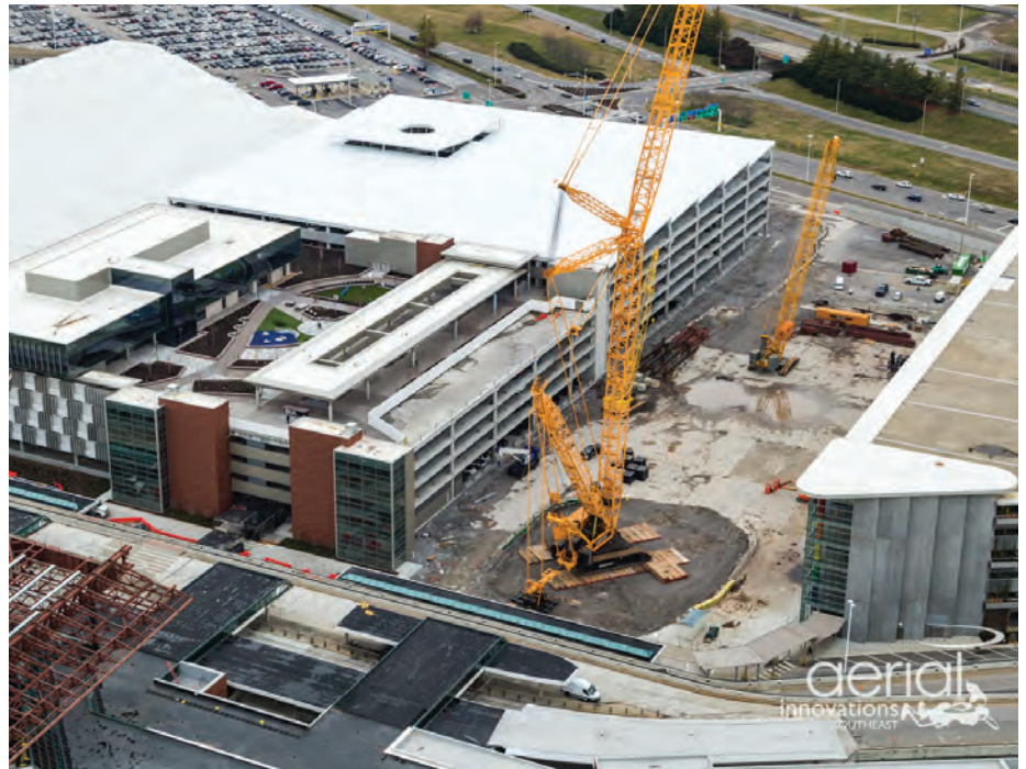
The new six-story garage was built in 18 months and opened in two stages.
