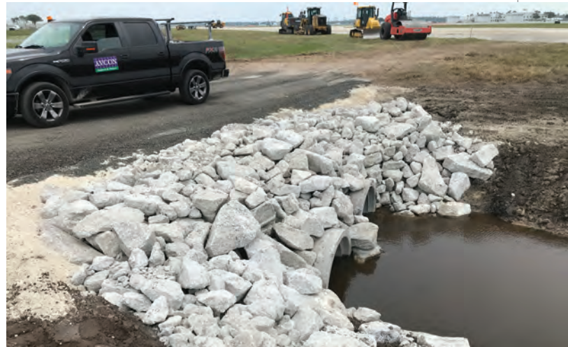
Temporary haul roads and staging areas helped expedite trips for construction vehicles.
