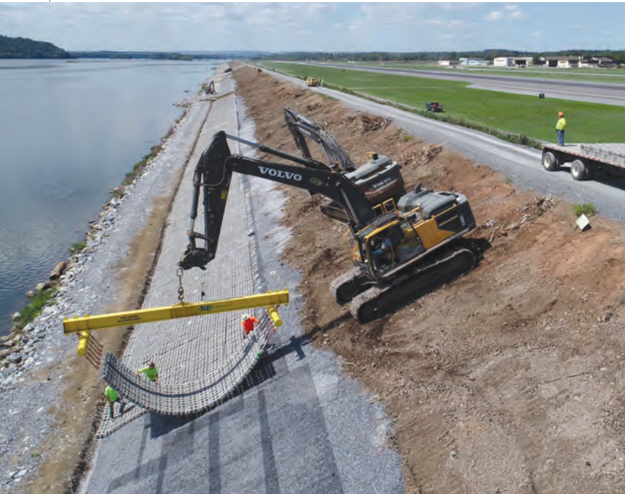
It took experienced equipment operators to work on the side and top of the levee.
