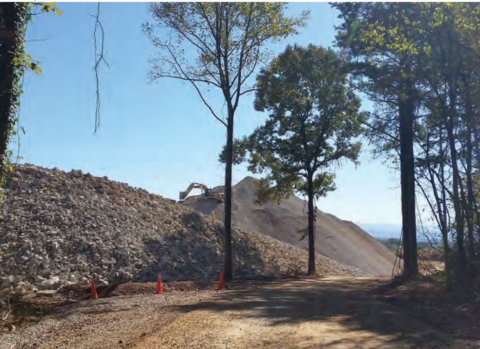
Crews moved more than 1 million cubic yards of earth during the project.
