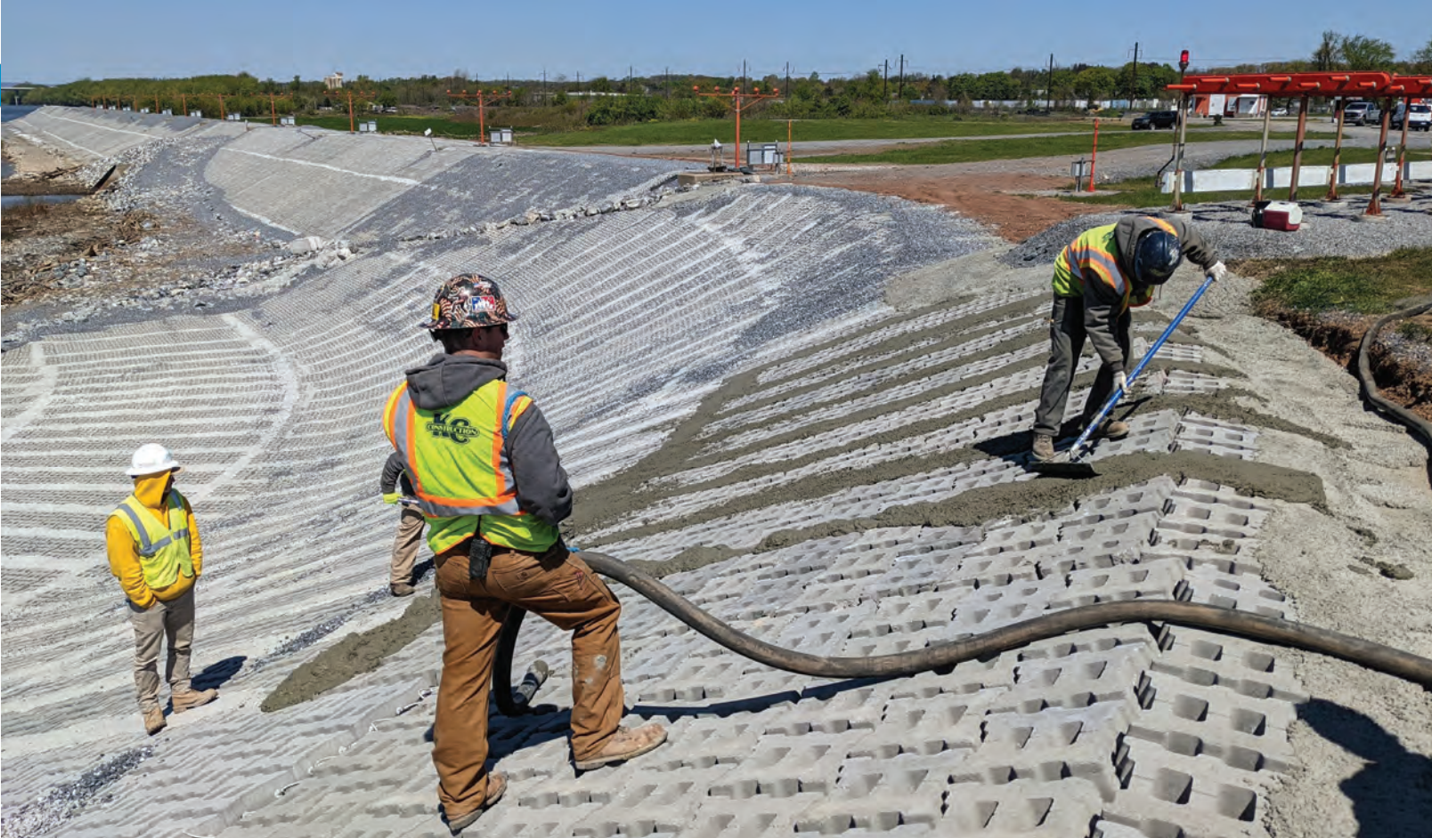
Workers placed concrete into the gaps between mats of articulated concrete blocks to help fuse them together.
