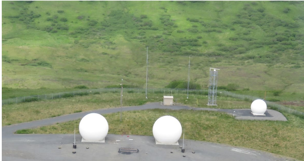
Figure 7-3: PSCA Telemetry Instrumentation Antennas with Radomes
