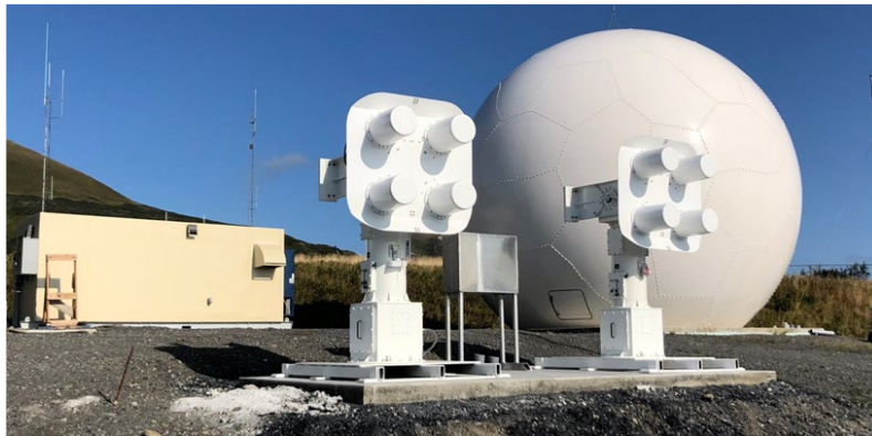
Figure 2-21: Instrumentation & Antenna Field
