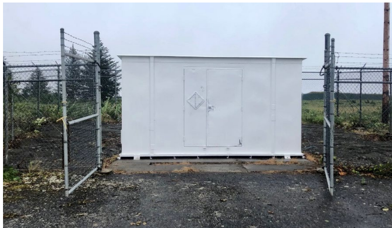
Figure 2-13: Hydrazine Storage Facility
