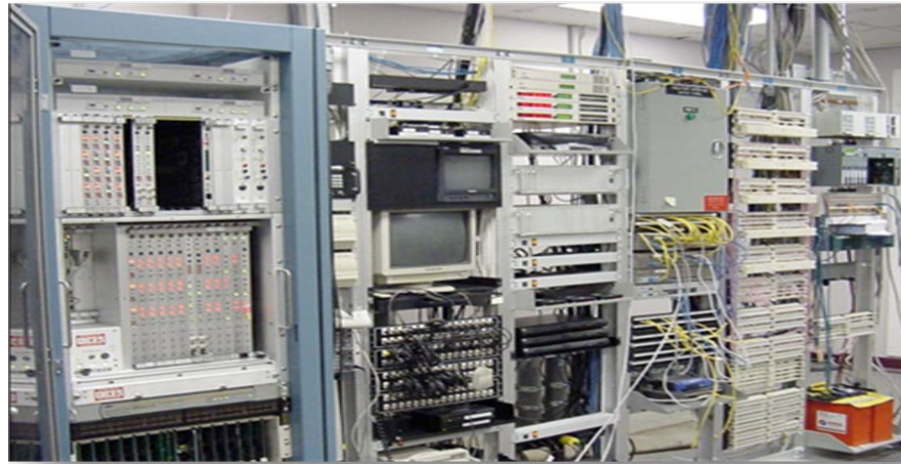
Figure 2-7: Typical Tech Control Equipment
