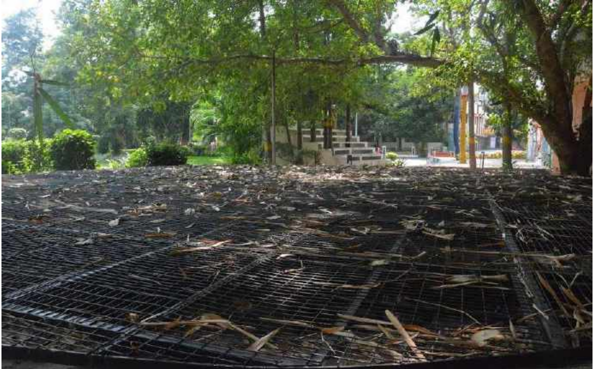
WELLS PROVIDED WITH MESH TO PREVENT THE DEBRIS ENTRY
