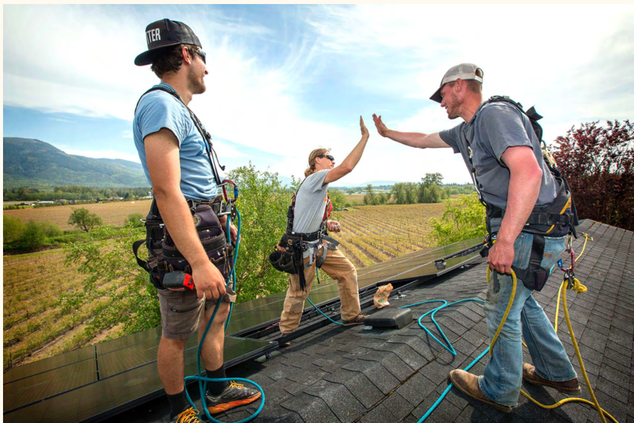
Sean Butenschoen of Probably Shouldn't Distillery and Ecotech Solar installer/Dean J. Koepfler
