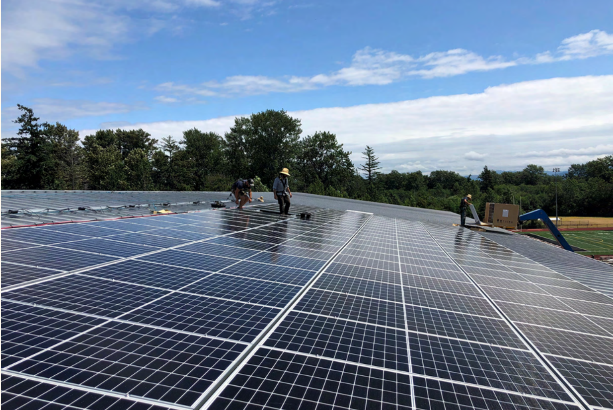
Solar installation on Lummi school/Spark Northwest
