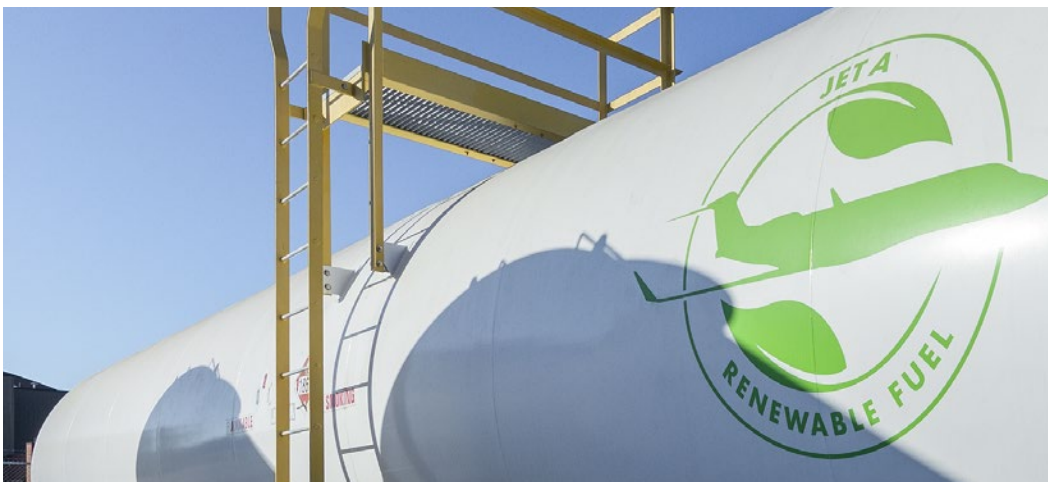
Sustainable aviation fuel tank
