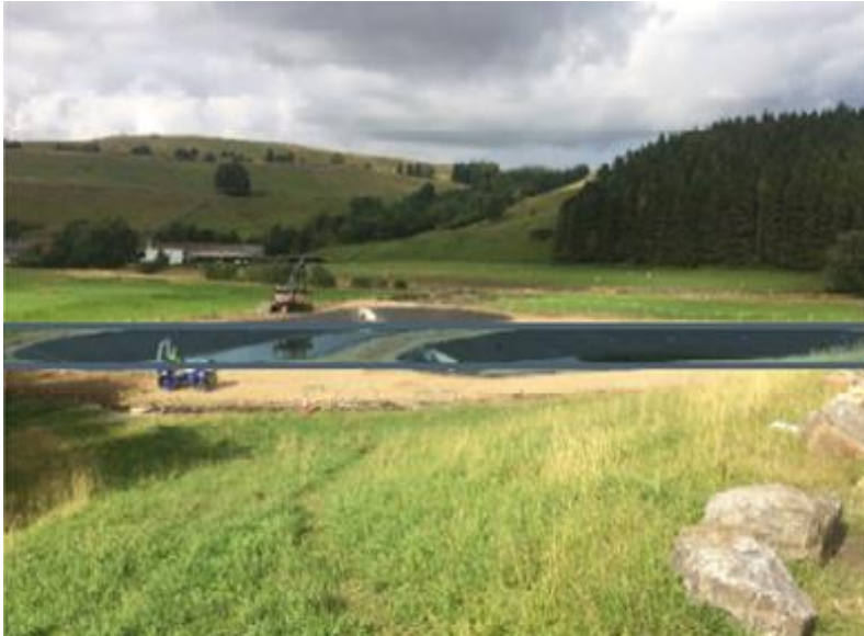
August 2022: Treatment ponds at Nent Hags with the new lining in waiting for the addition of natural treatment media.
