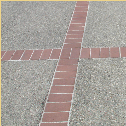
Example of plaza paving consisting of exposed aggregate concrete with brick bands (2003).
