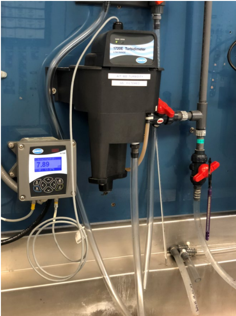
In-line Water Quality Meters at the Maplewood WTP
