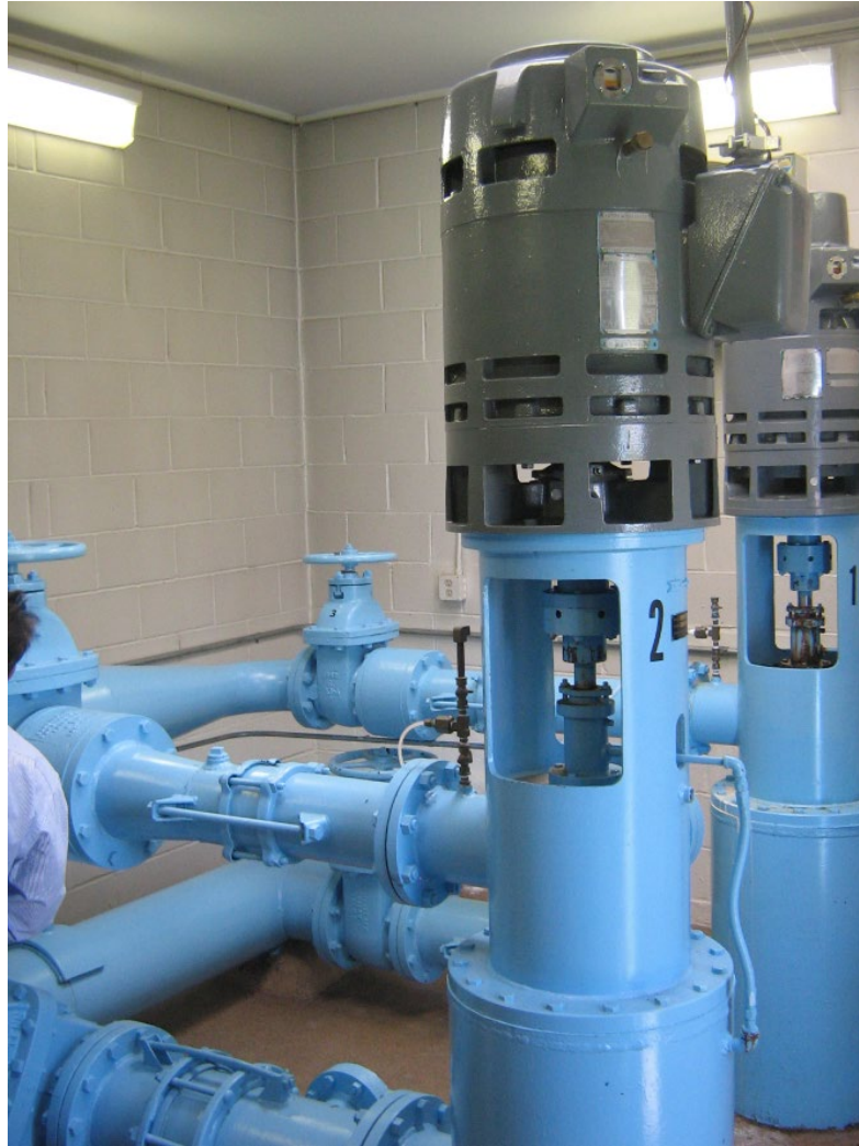
Tiffany Park Booster Pump Station
