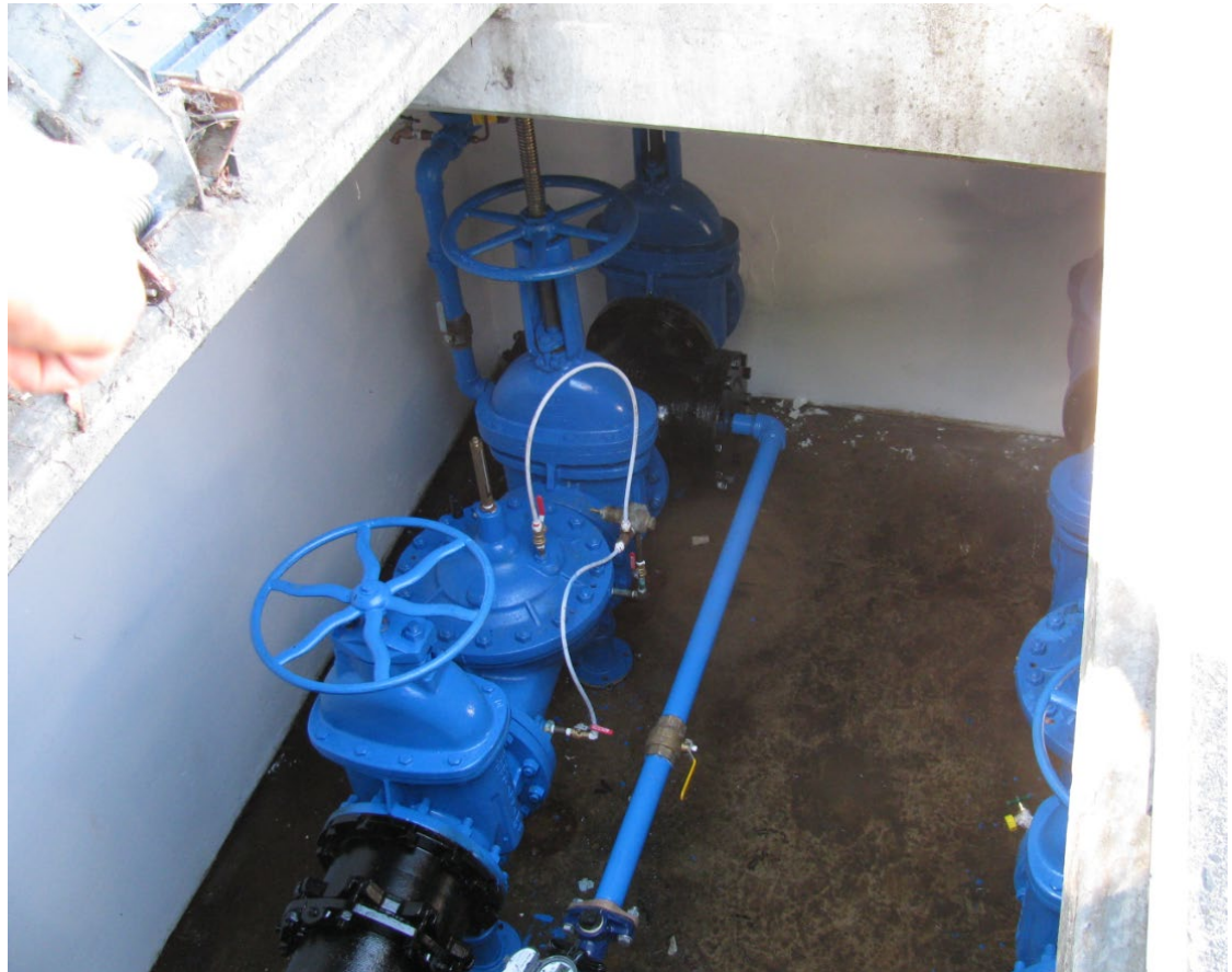
Pressure Reducing Valve (PRV) 52
