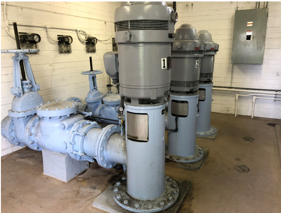
Highlands Booster Pump Station
