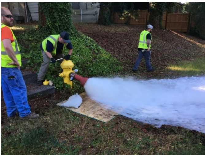
Fire Hydrant Test – June 2018
