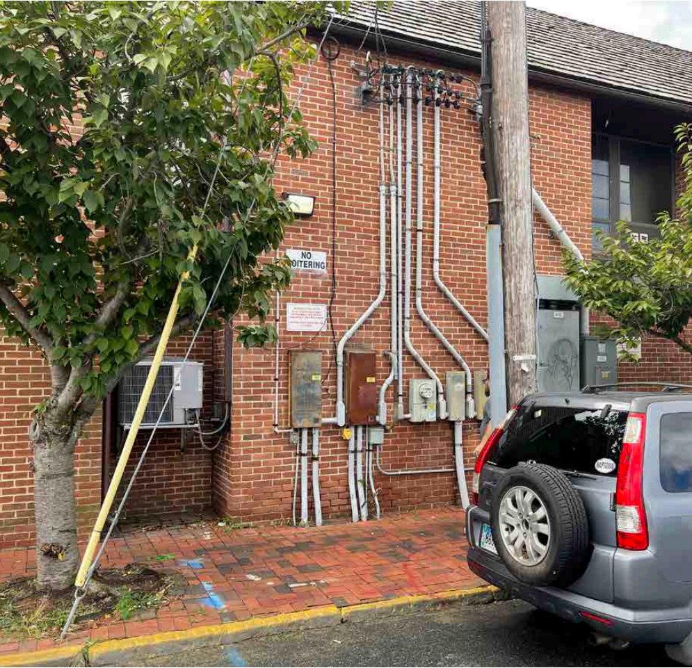
Existing Electrical Service Equipment on Harbormaster Office
