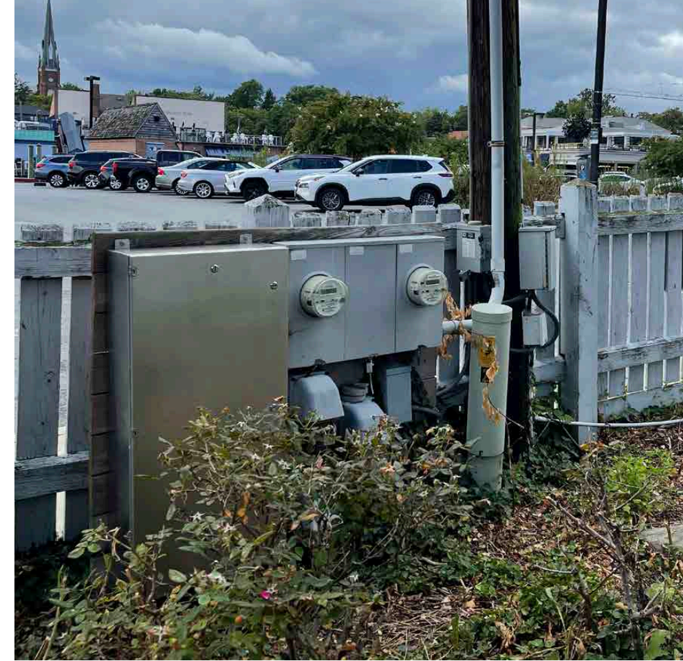
Existing Electrical Service Equipment at Burtis House Fence
