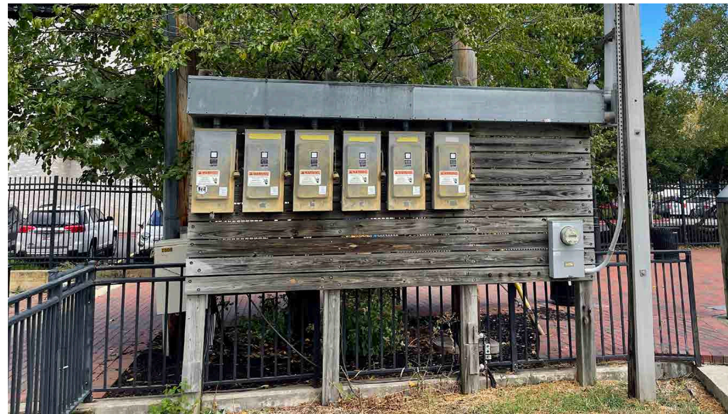
Existing Electrical Service Equipment at Burtis House Waterside
