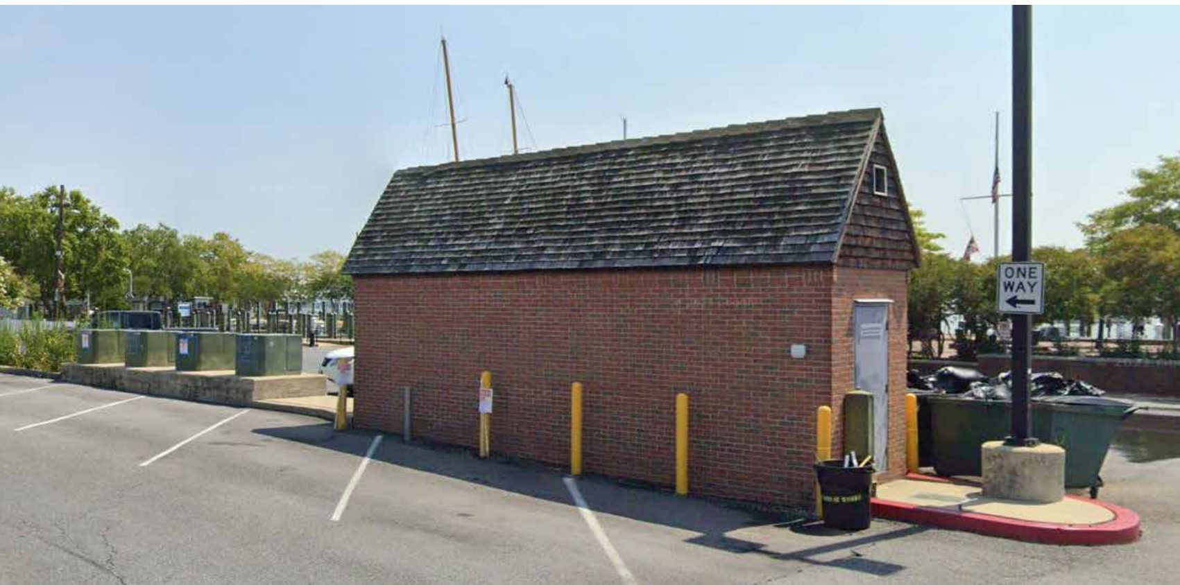
Existing Electrical Building ("Birdhouse") and Exterior Ground-Mounted Transformers
