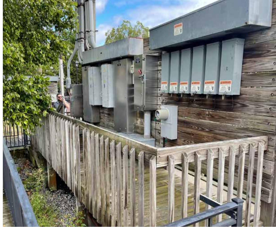
Existing Electrical Service Equipment at Burtis House Waterside
