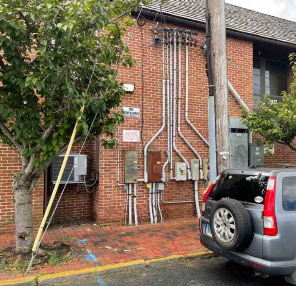
Existing Electrical Service Equipment on Harbormaster Office
