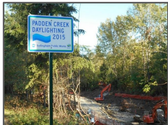
The Padden Creek daylighting project will improve creek conditions for salmon and other wildlife.
