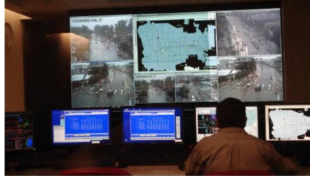
Figure 5-3 – Pasadena Traffic Management Center
