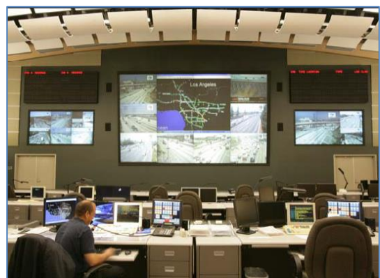
Figure 5-1 – Los Angeles Regional Transportation Management Center
