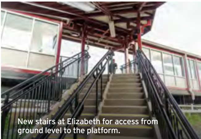
Sections of new platforms continued to open in FY2022 on the Elizabeth Station rehabilitation project.
