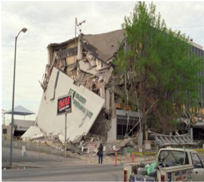
Figure 2-7. The Kaiser Permanente Office Building, a non-ductile concrete building that suffered partial collapse in the January 17, 1994 Northridge earthquake.
