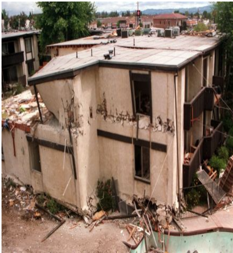
Figure 2-5. The Northridge Meadows Apartments after the January 17, 1994 Northridge earthquake. Source: Los Angeles Times
