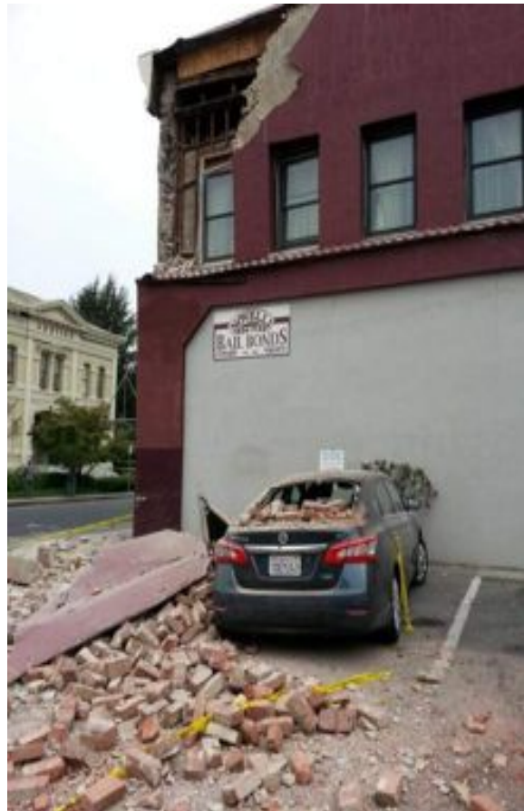
Figure 2-4. Damage to an unretrofitted URM building in the 2014 South Napa earthquake. Adjacent buildings were temporarily closed until this building could be secured. Photo: J. Maffei
