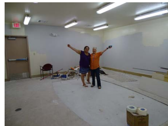
Top, Enrollment Clerk Chris Miller working on moving files into the new filing room. Bottom, construction in progress. Photos courtesy Leslie Fall-Leaf and Dana Murrell.
