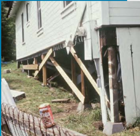
This home's pier-and-post foundation was damaged during an earthquake. The diagonal bracing was added after the earthquake to temporarily stabilize the home during repairs.
