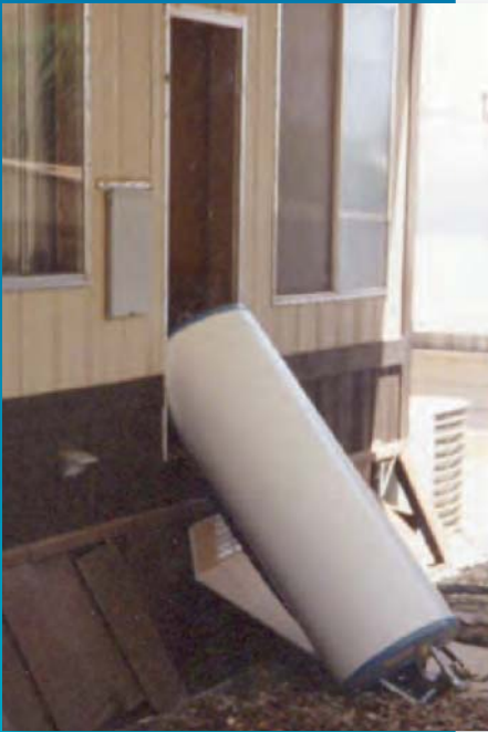
During an earthquake, an unbraced water heater can topple, which can start a fire or lead to major water damage.
