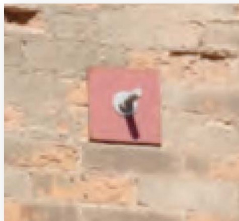
A steel plate with anchor bolts.
