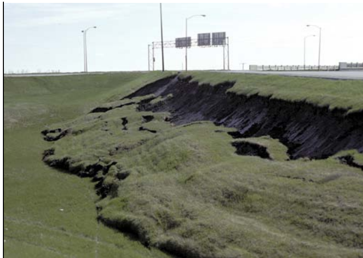
FIGURE 34 SEDIMENT SLUMPING IN THE RED RIVER VALLEY
