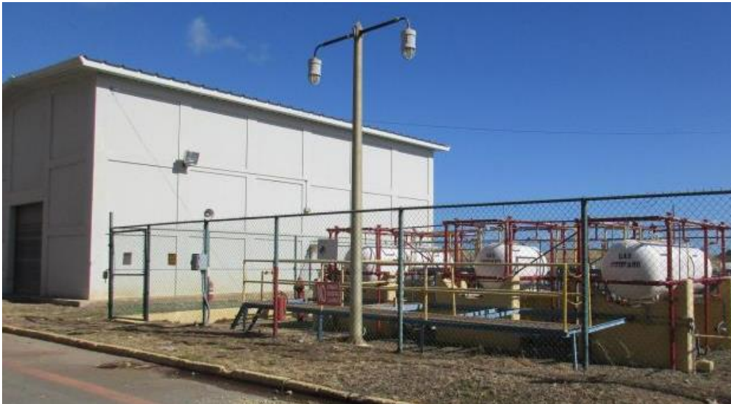
Temperature- and humidity-controlled storage building on the left for spare motors and other parts. Propane tanks on the right.
