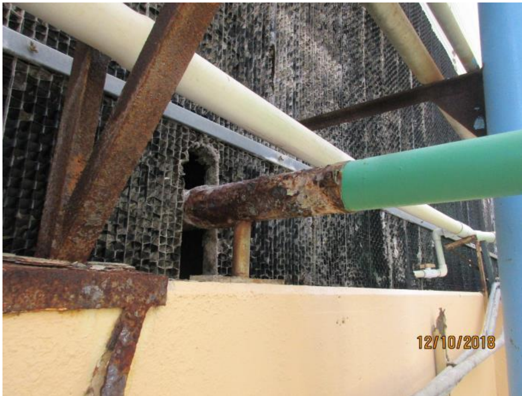
Figure 3-5 — Cooling Tower Corrosion, Units 5 and 6
