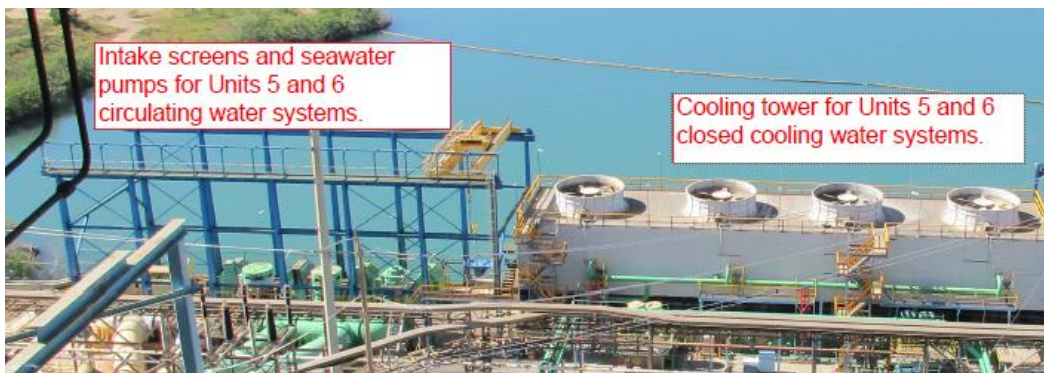
Figure 2-3 — Units 5 and 6 Seawater Intake and Closed Cooling Tower
