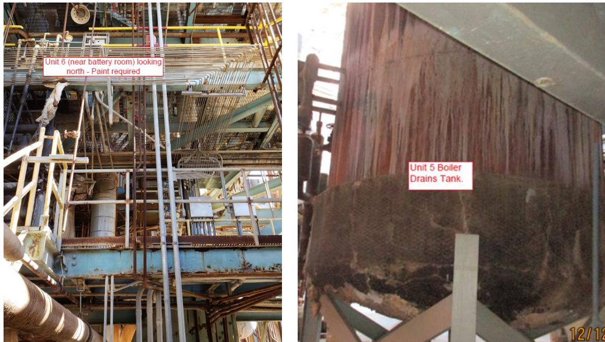
Figure 3-4 — Corrosion Examples, Units 5 and 6
