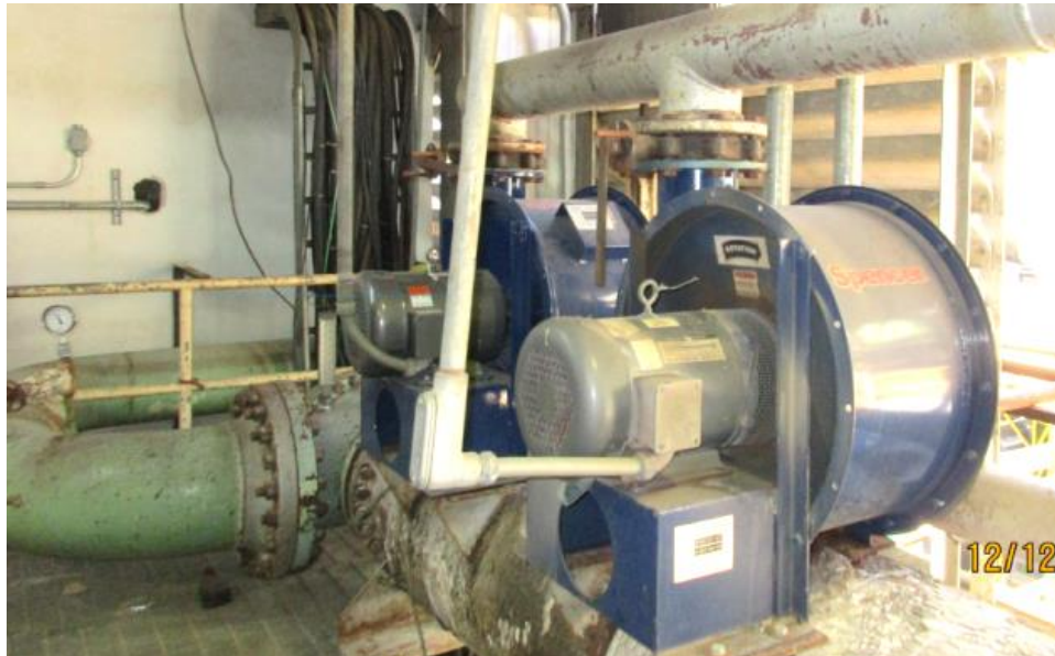
Figure 3-2 — Gland Steam Exhauster Blowers
