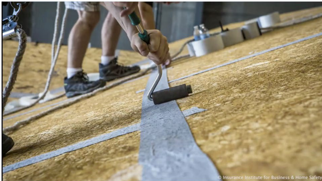
Figure 3. Installing a sealed roof deck system; taping the seams of roof sheathing.
