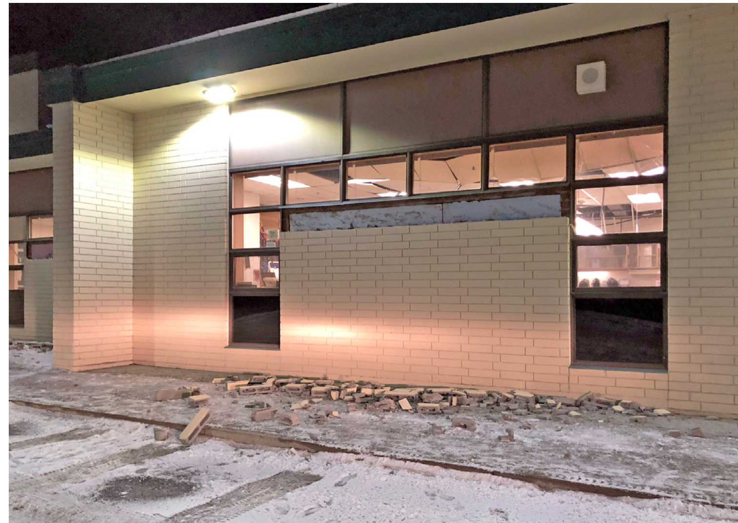
Significant wallboard cracking, brick and masonry veneer damage, window damage, and cladding damage caused falling hazards. – Elementary School Fallen Brick Veneer. Credit: David Stierwalt, Reid Middleton, Inc.
