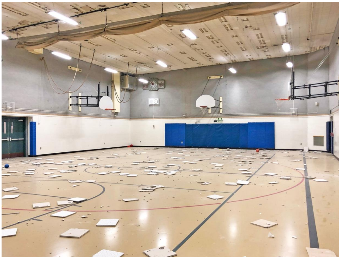
Figure 2.2-1. Nonstructural Ceiling Tile Earthquake Damage to an Elementary School in Eagle River, Alaska, from the 2018 M7.0 Anchorage Earthquake (Photo by Reid Middleton, Inc.).
