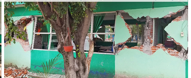
Primary school wall failure due to diagonal tension in unreinforced masonry bearing wall
