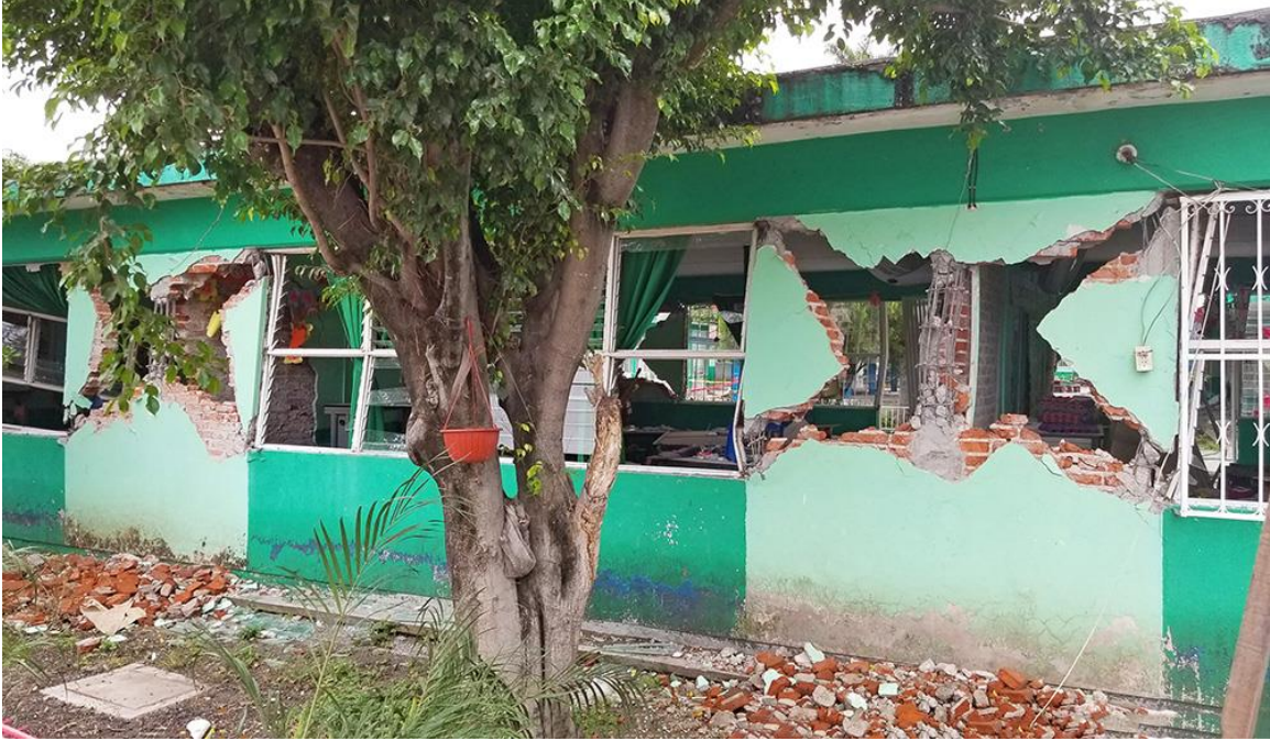
Figure 3.1.3-1. Structural Earthquake Damage to a Primary School in Central Mexico from the 2017 M7.1 Central Mexico Earthquake (Photo by Reid Middleton).
