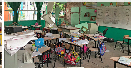
Primary school unreinforced masonry infill walls damage
