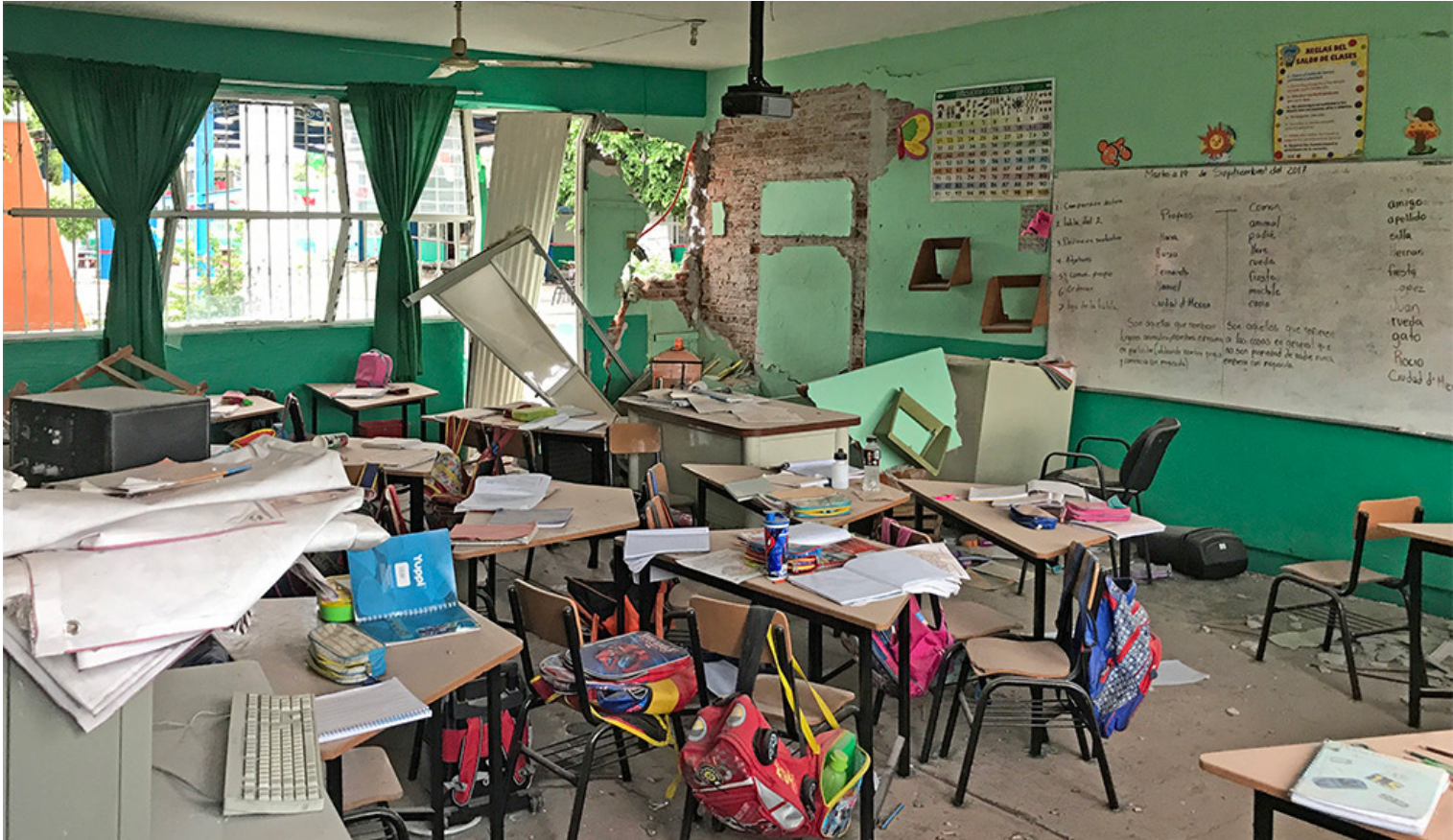
Damaged Primary School in Jojutla. The unreinforced masonry infill walls were damaged. Many Washington state schools are constructed similarly. Credit: Erik Bishop, Reid Middleton, Inc.
