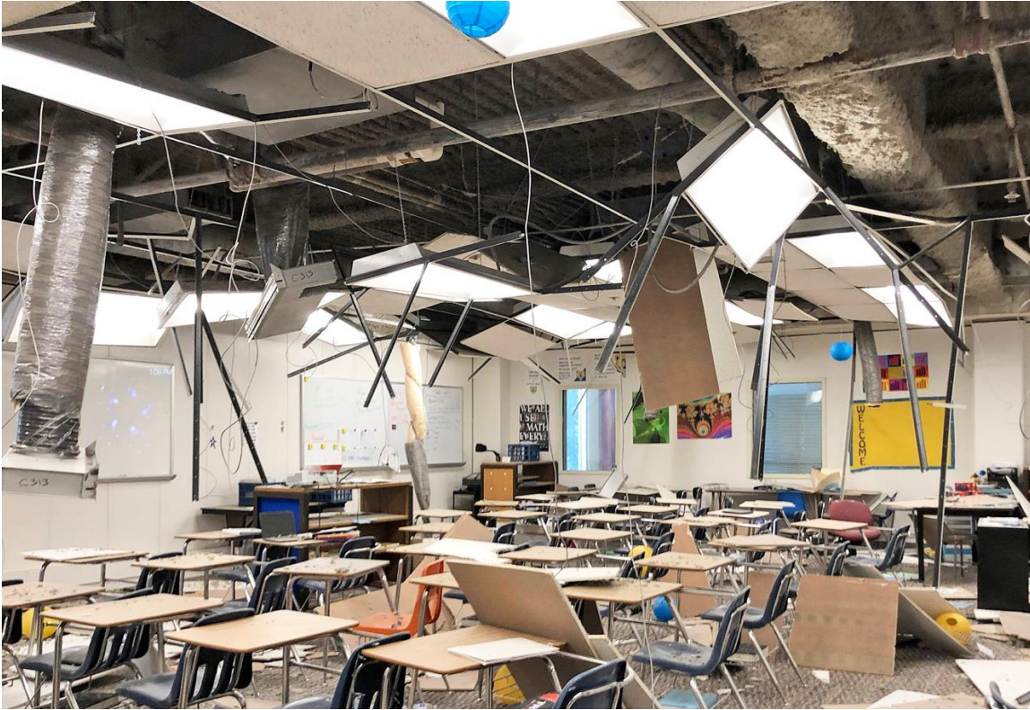
Figure 3.1.5-1. Nonstructural Earthquake Damage to a High School in Anchorage, Alaska, from the 2018 M7.0 Anchorage Earthquake (Photo by Reid Middleton, Inc.).
