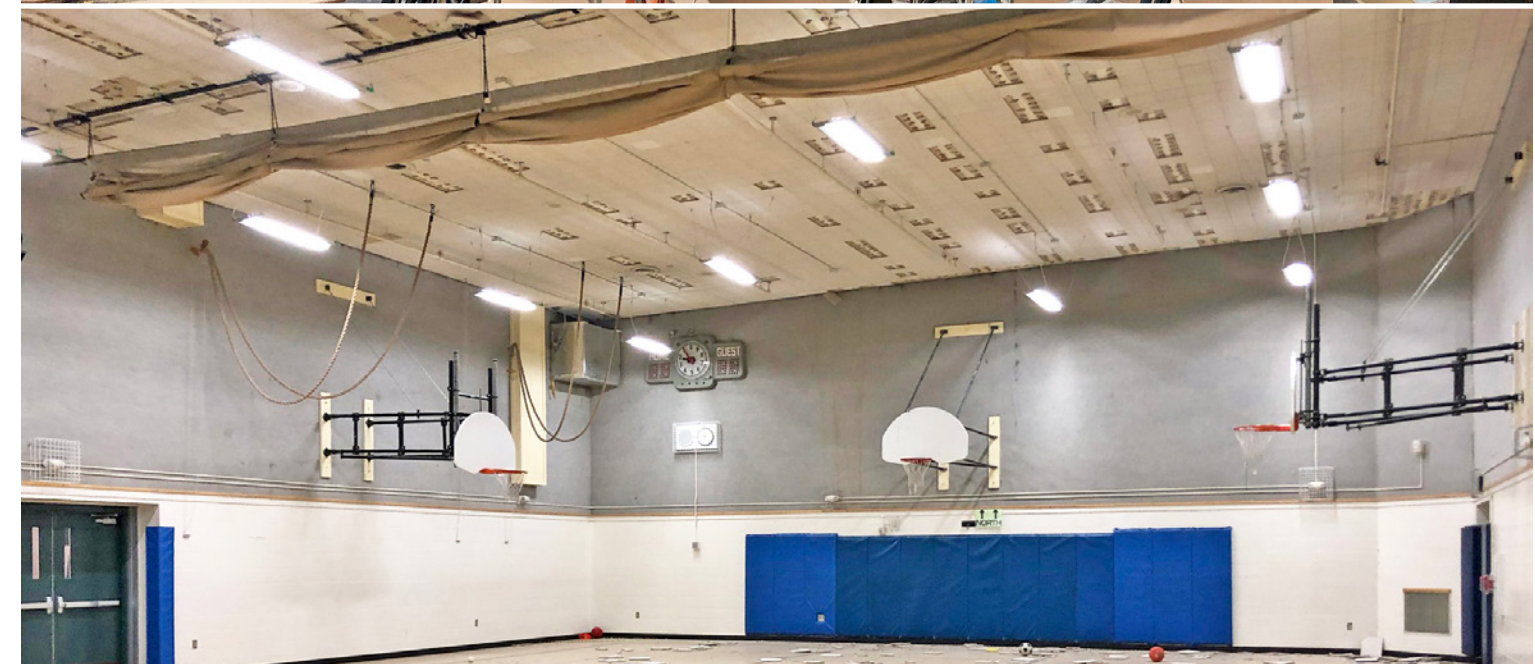
Extensive ceiling system damage in many schools caused falling hazards during and after the earthquake. Credit: David Stierwalt, Reid Middleton, Inc.
