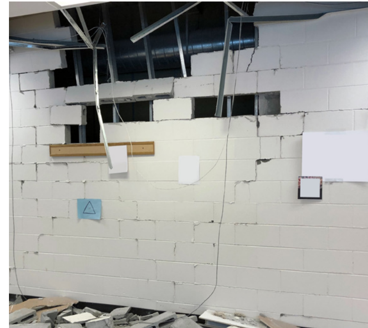
Considerable cracking and damage in CMU bearing and partition walls. – High School CMU Partition Wall Damage. Credit: David Stierwalt, Reid Middleton, Inc.
