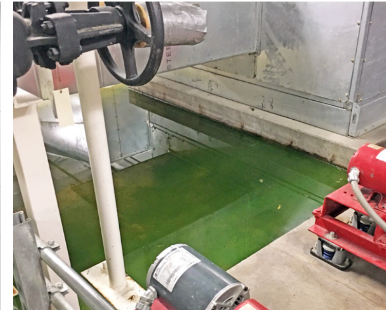
Some suspended and ground supported HVAC and mechanical equipment sustained damage and sheared their support structural bolts causing unsafe conditions and chemical leaks. – Elementary School Leaking Glycol in Fan Room. Credit: David Stierwalt, Reid Middleton, Inc.
