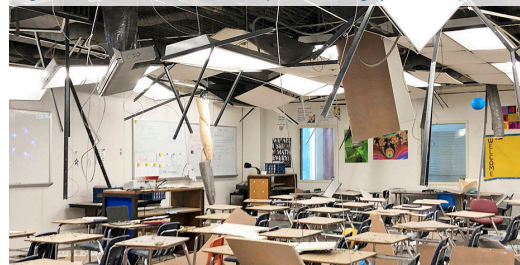
High school classroom extensive suspended ceiling system collapse
