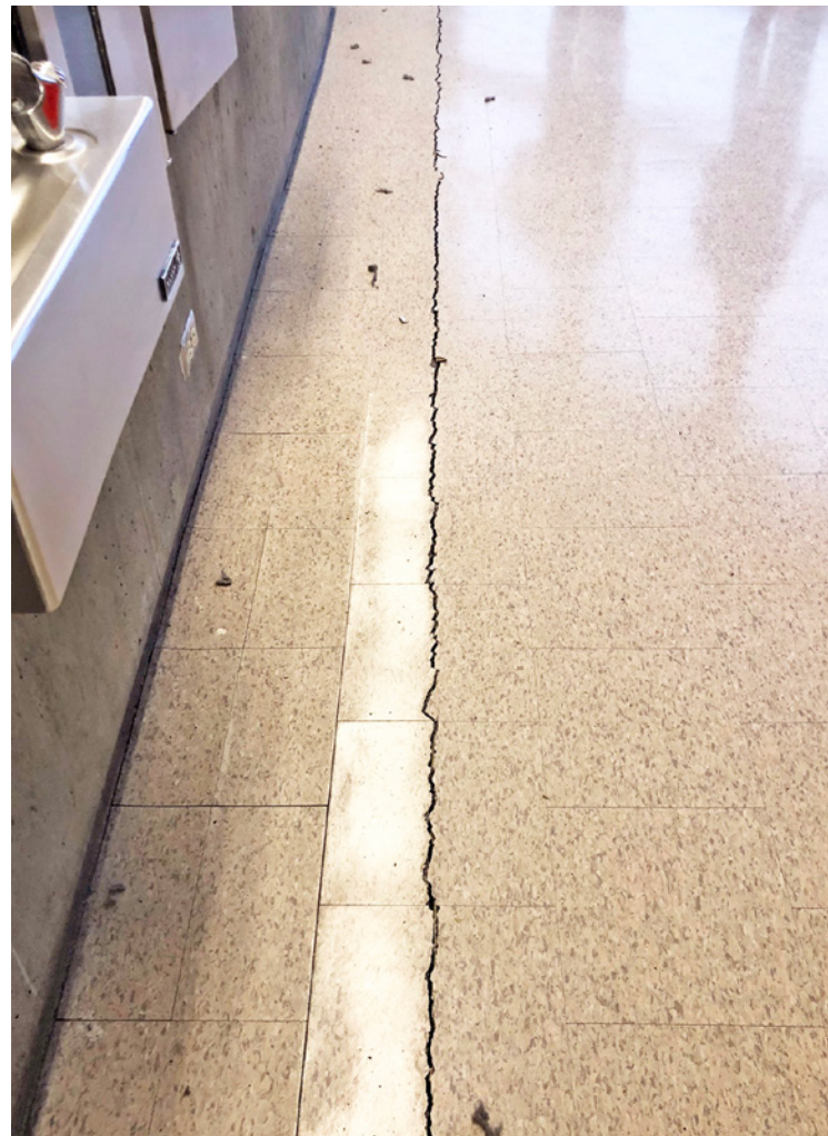
Floor and floor finish cracking. – High School Flooring Crack. Credit: David Stierwalt, Reid Middleton, Inc.
