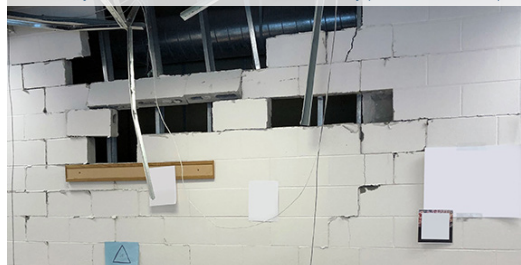
Elementary school unreinforced concrete masonry partition wall collapse
