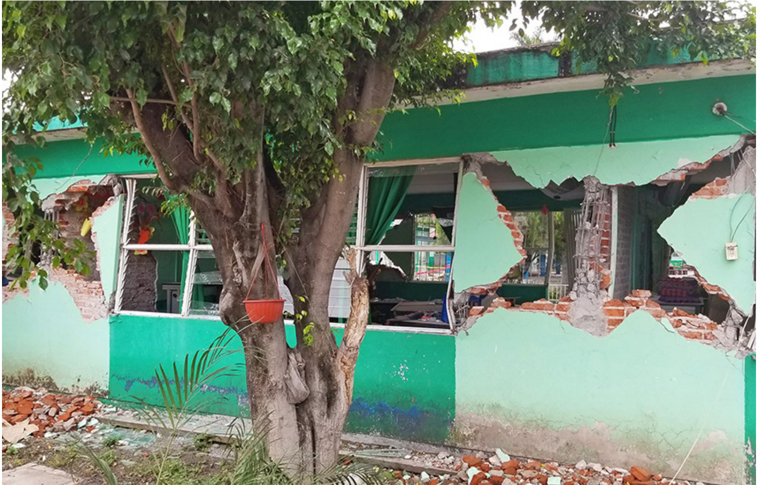
Damaged Primary School in Jojutla. Total failure due to diagonal tension in unreinforced masonry wall. Many Washington state schools are constructed similarly. Credit: Erik Bishop, Reid Middleton, Inc.
