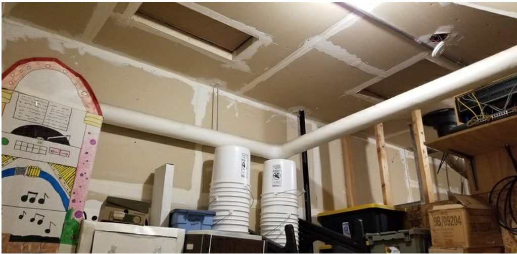
Figure 1-10. Fall prone items in second floor storage area
