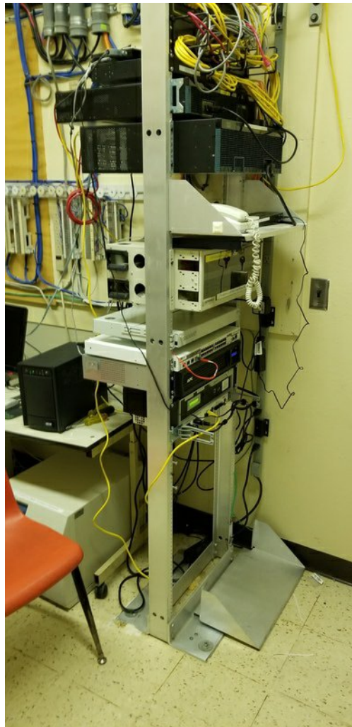
Figure 1-8. Fall prone content and shelving that is not adequately braced
