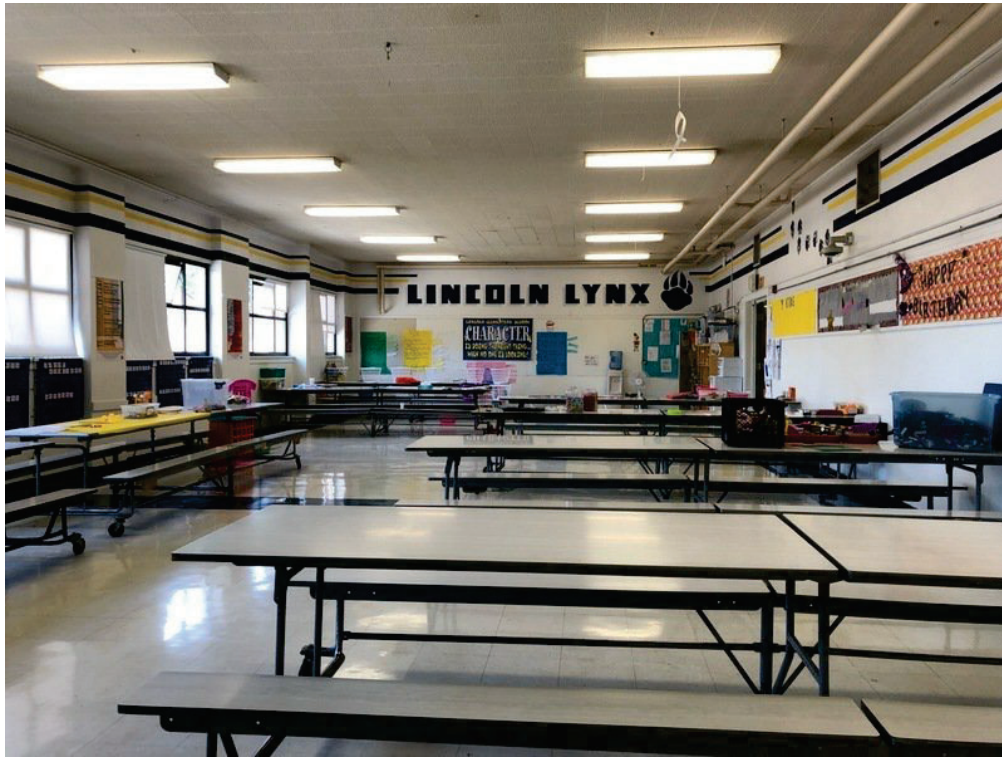
Figure 1-3. Lunchroom. Note hard ceiling, surface mounted light fixtures, with exposed unbraced plumbing and fire protection piping.
