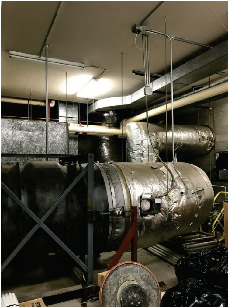
Figure 1-10. Classroom building mechanical space
