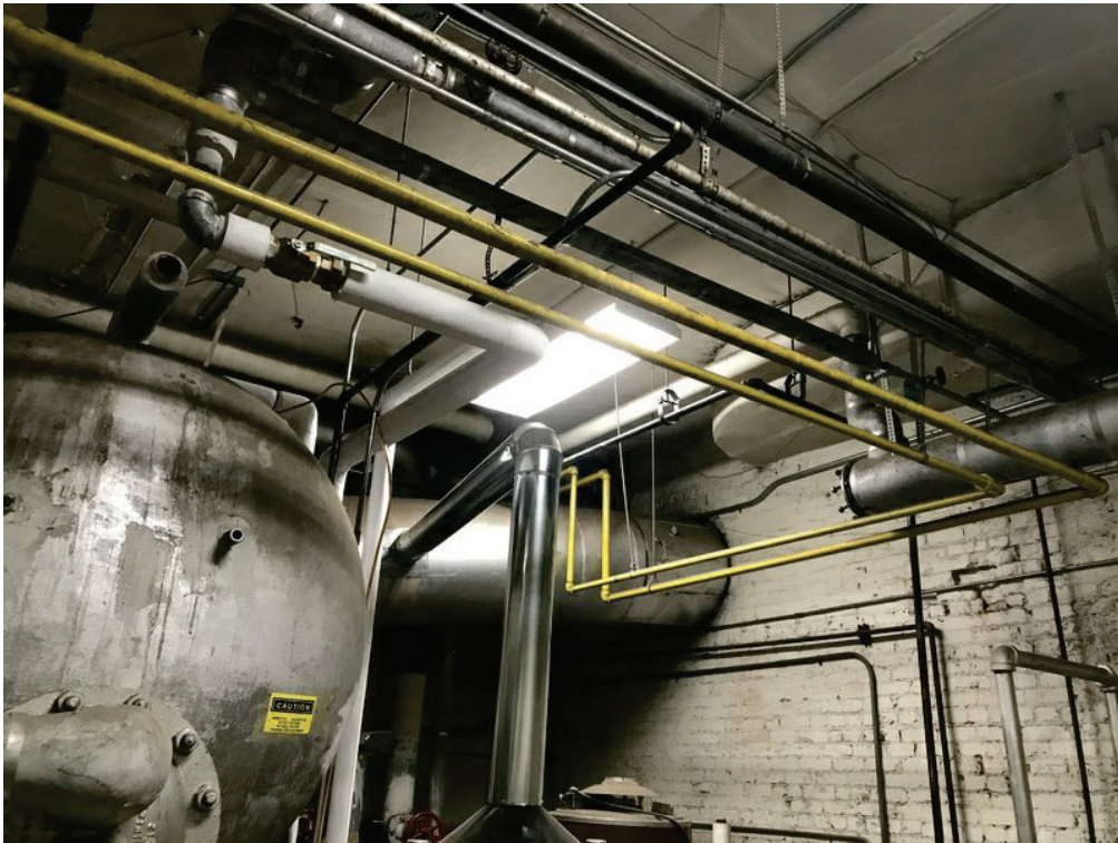
Figure 1-2. Mech Room - gas piping is painted yellow
