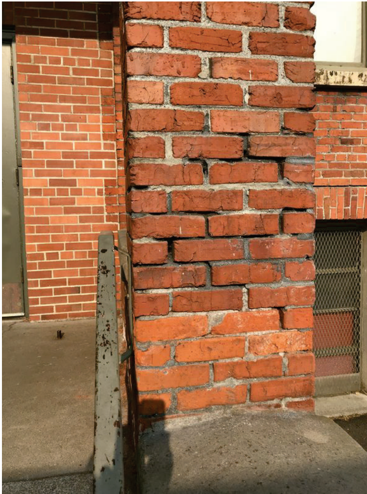
Figure 1-5. Deteriorated mortar in masonry column at east entry
