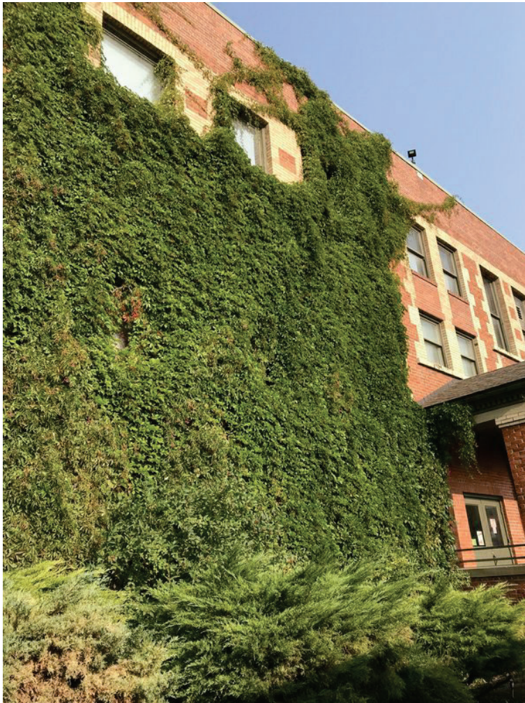
Figure 1-6. Ivy growth on east wall of building
