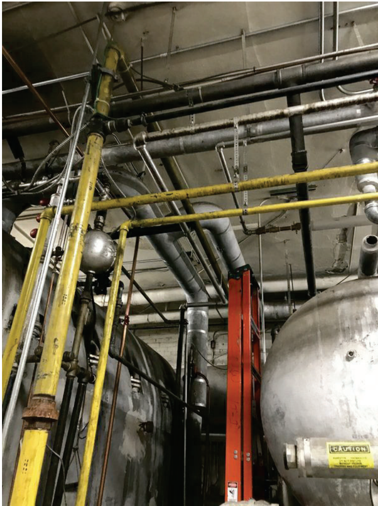
Figure 1-3. Mech Room - gas piping is painted yellow
