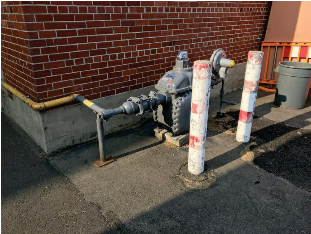
Figure 1-7. Gas meter at northwest corner of building
