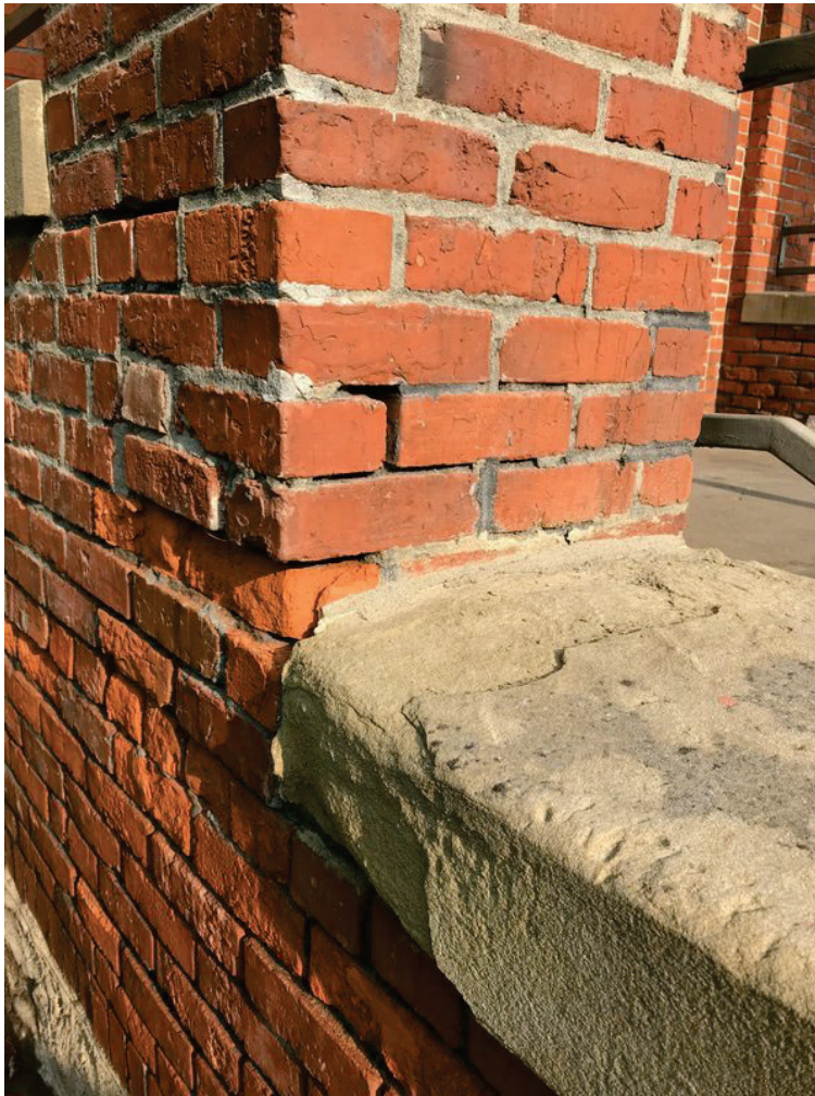
Figure 1-4. Deteriorated mortar in masonry column at east entry
