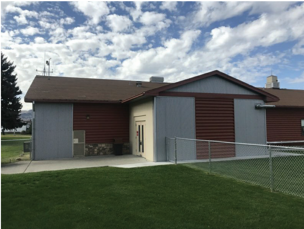
Figure 1-8. Exterior view of building from the northeast & facing south; showing the west end of the classroom wing.
