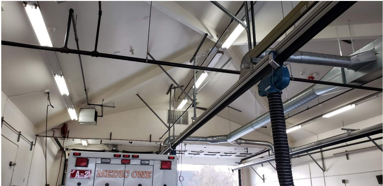
Figure 1-6. Everett Fire Station 2, Apparatus Bay Overhead Door Support
