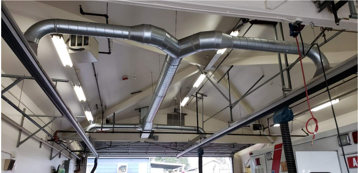
Figure 1-5. Everett Fire Station 2, Ductwork at Apparatus Bay Ceiling
