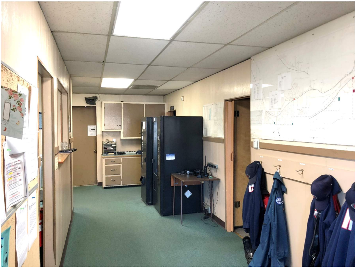
Figure 1-9. Upstairs Hallway with Unbraced Tall, Narrow Contents – Typical Throughout
