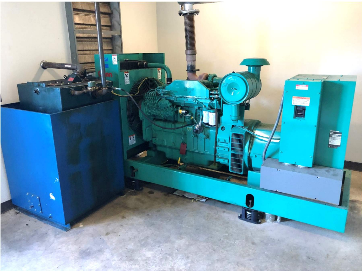
Figure 1-10. Unbraced Mechanical Equipment
