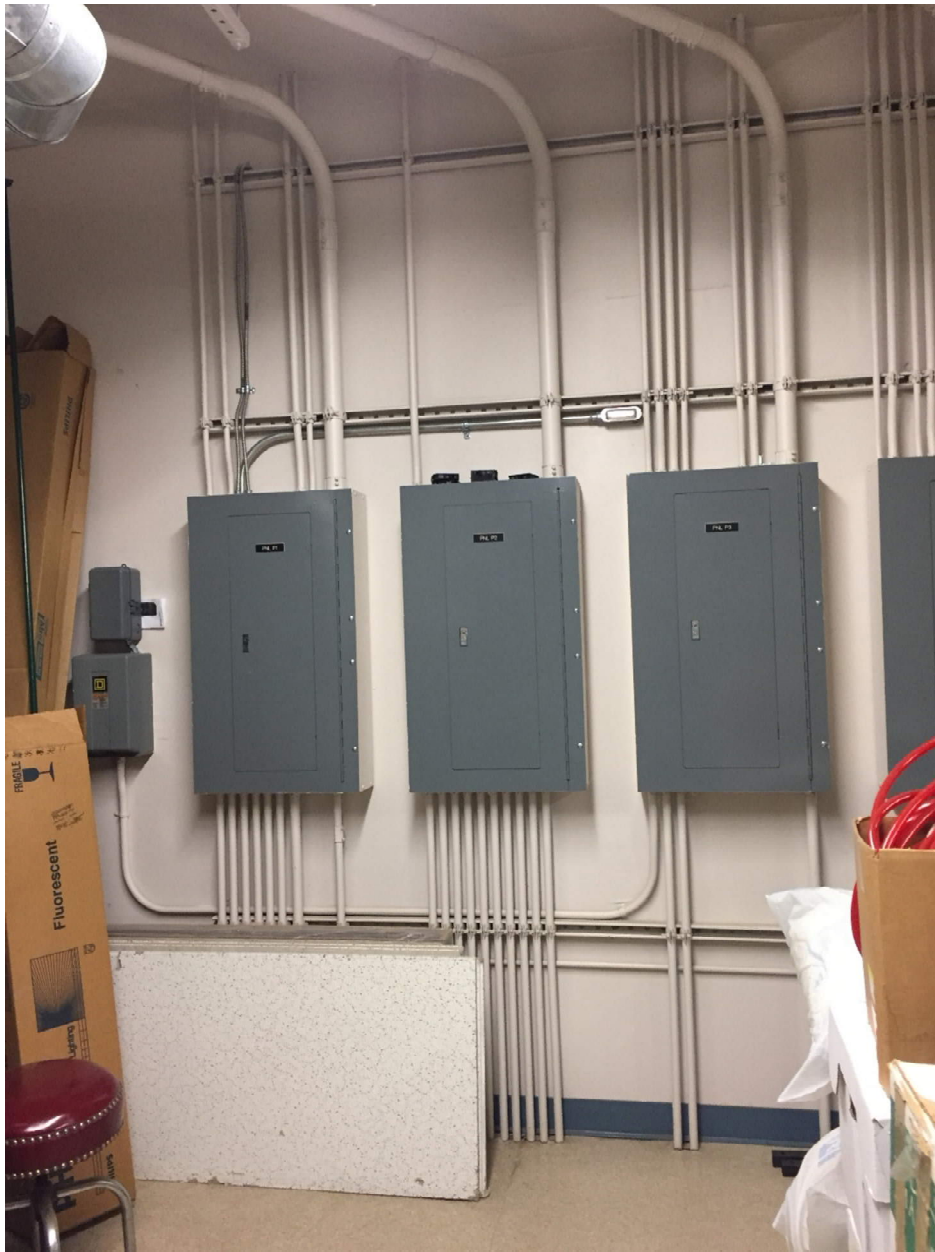
Figure 1-9. Walla Walla Station 41, Electrical Room
