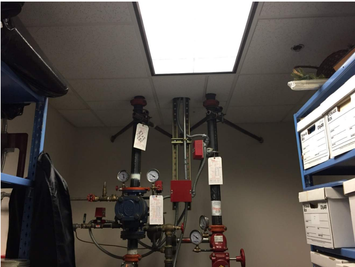
Figure 1-6. Walla Walla Station 41, Mechanical Room
