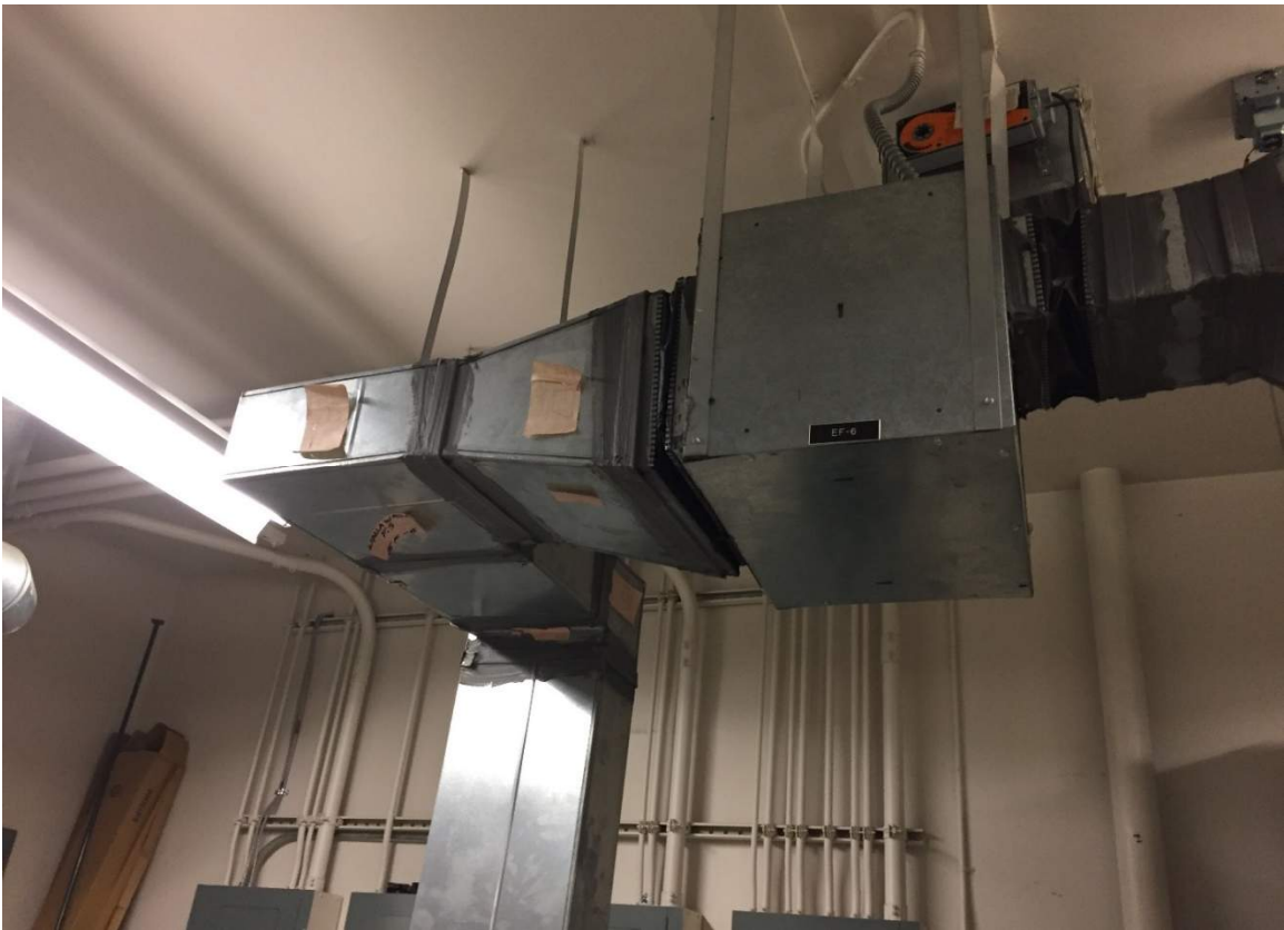
Figure 1-7. Walla Walla Station 41, Overhead Ductwork
