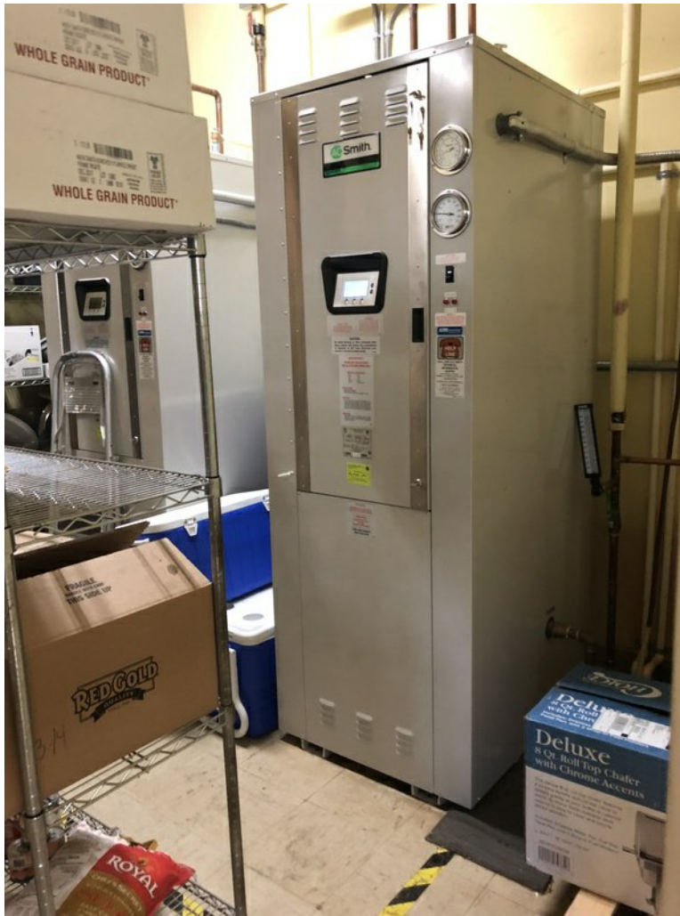
Figure 1-10. Tall Unbraced Nonstructural Components, Typical Throughout
