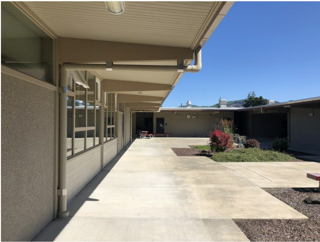
Figure 1-9. Roof Overhang Framing Condition
