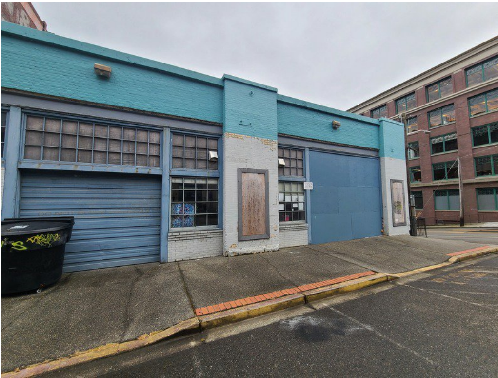
Figure 1-1. The west side of the building. Some minor deterioration is present at the URM walls.
