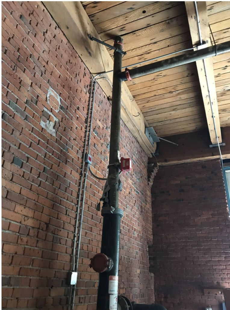
Figure 1-6. Northeast corner of the building on the first floor. Appears to be minor damage to the URM, as is common in various locations throughout the building.
