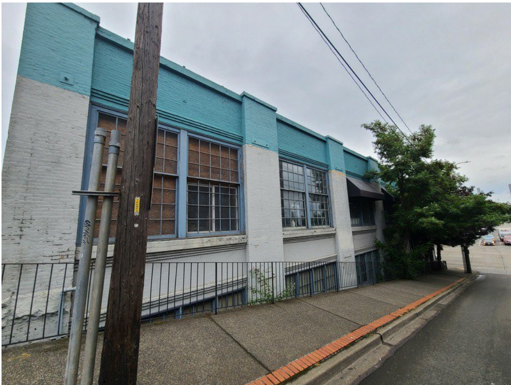
Figure 1-2. The south side of the building. Some minor deterioration is present at the URM walls
