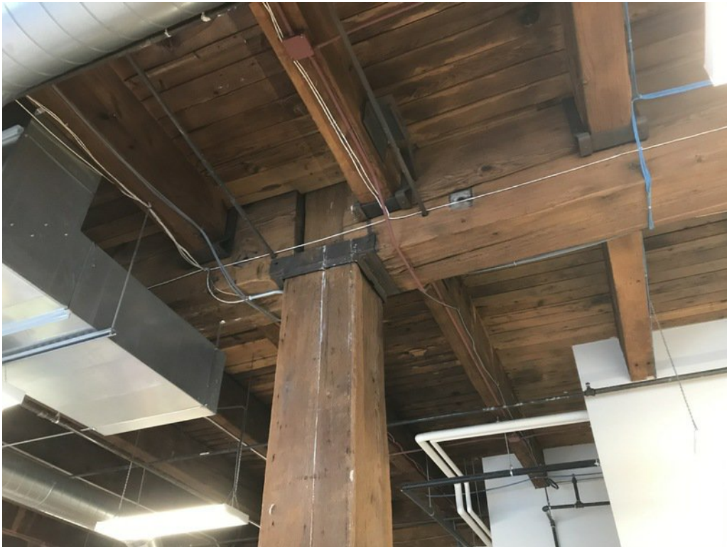
Figure 1-5. Wood post to girder connection. Some minor splitting is present in the girder.
