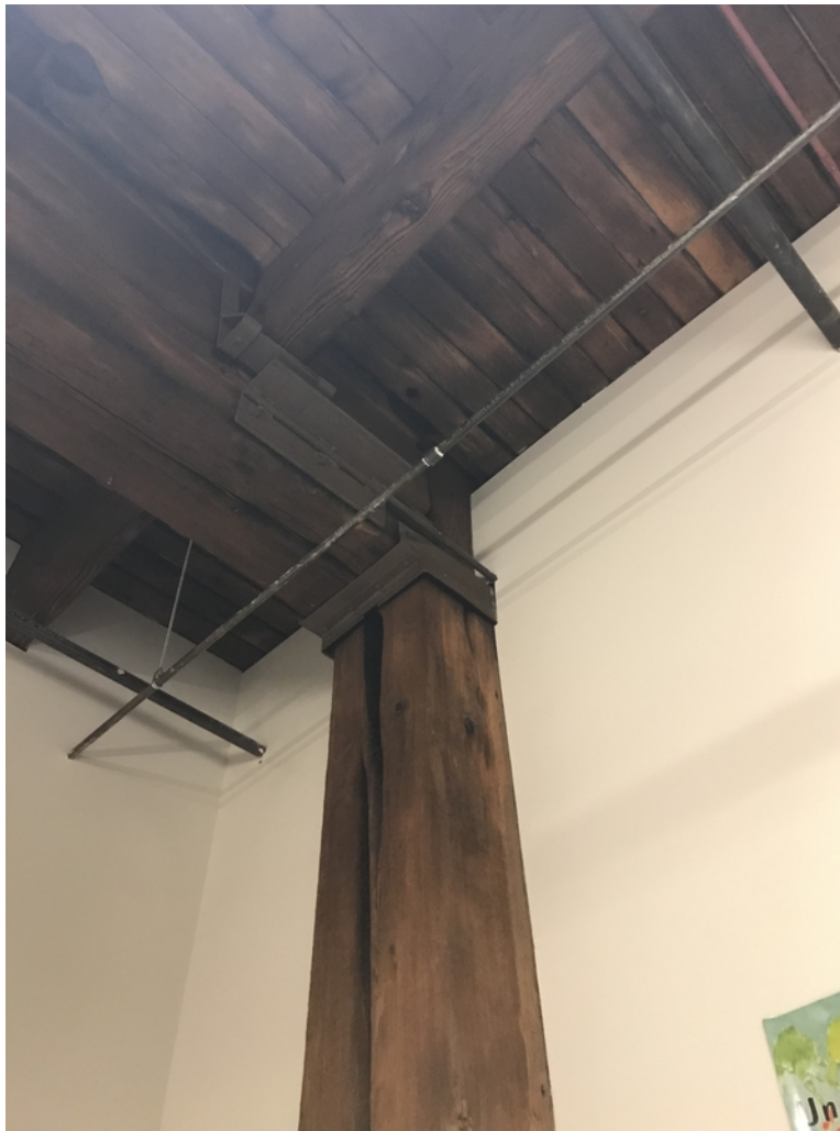
Figure 1-3. Wood post supporting a girder at a partition wall. Post has major split, and girder has minor split where it bears on the post.
