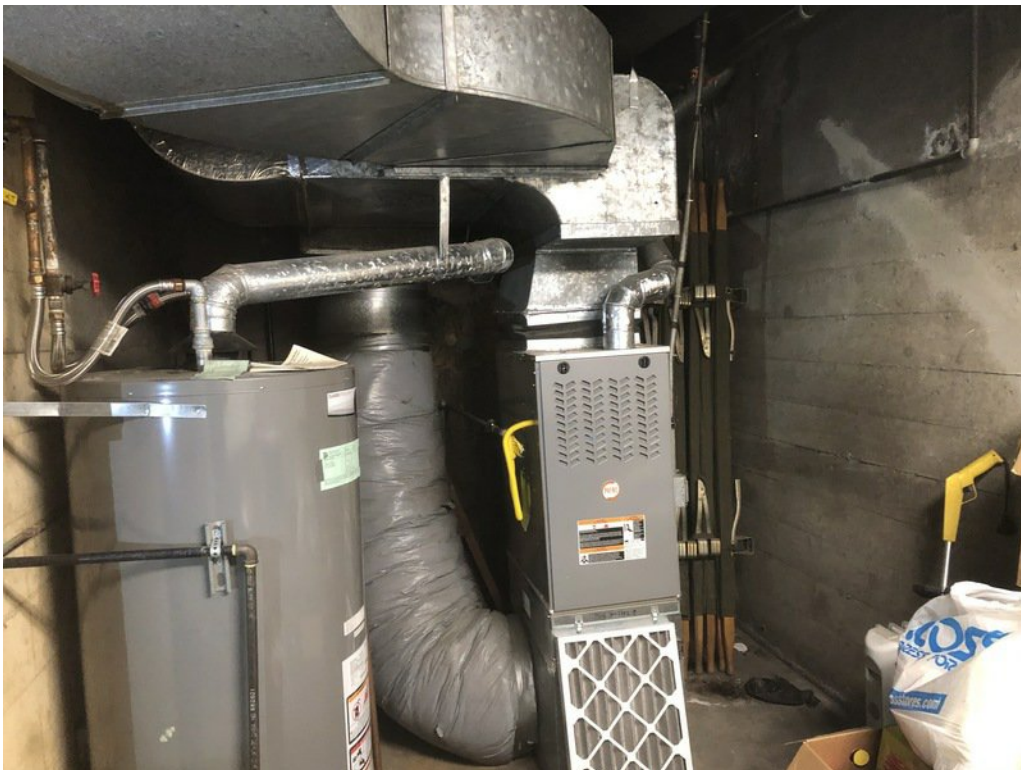
Figure 1-8. Figure-8 Mechanical Units in Basement
