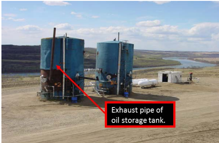
Figure 179. Oil storage tanks and exhaust pipe.
