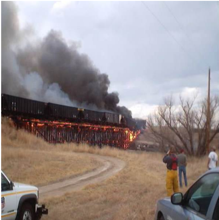
Figure 114. Railroad trestle fire.
