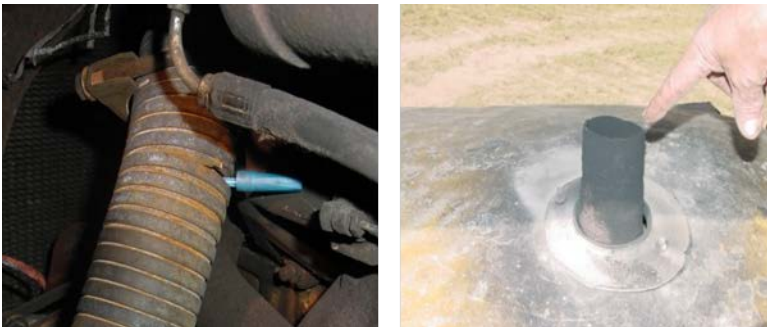
Figure 104. Damaged exhaust systems.
