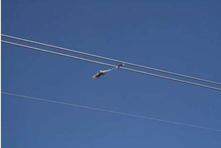
Figure 131. Mylar balloon stuck on transmission lines.
