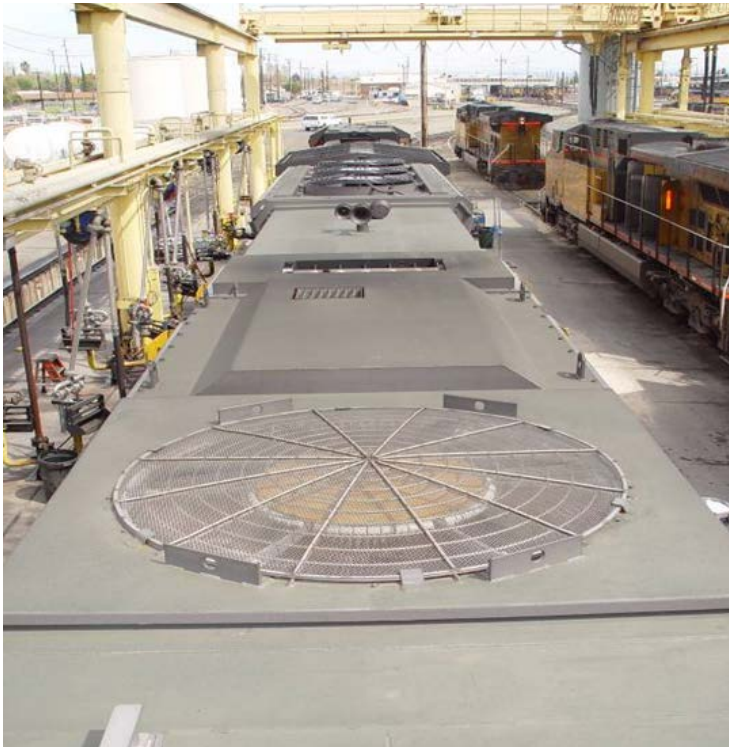
Figure 121. Dynamic brake grid exhaust outlet.
