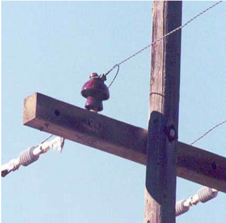
Figure 137. Typical crossarm insulator on a wooden mounting peg.
