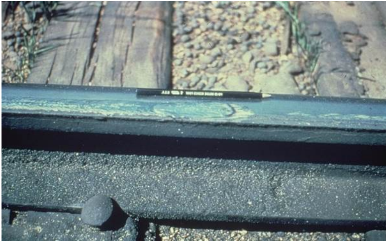
Figure 124. Train wheel slip on train track.
