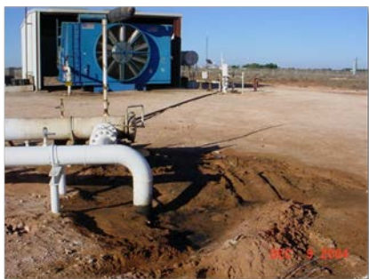
Figure 92: Natural gas compressor station
