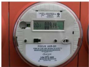
Figure 33: Oncor smart meter
