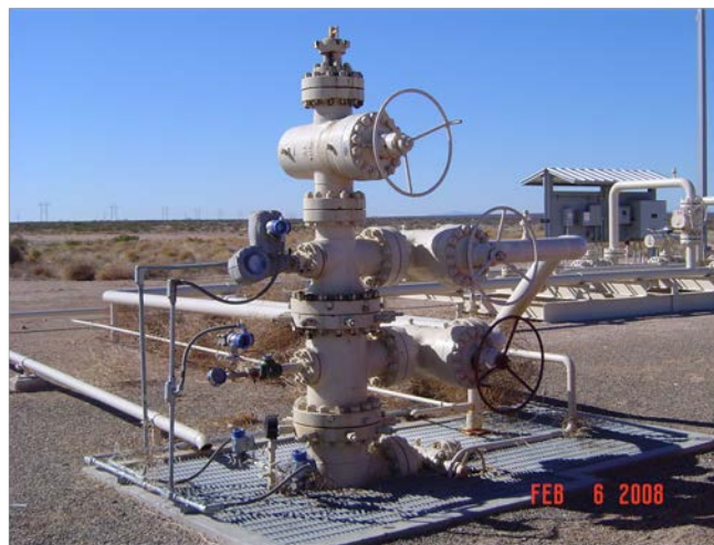
Figure 79: Gas well and meter run delivering to intrastate pipeline.
