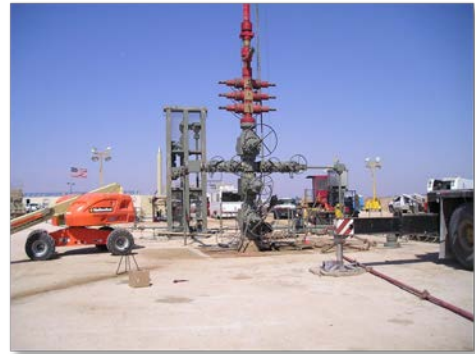
Figure 93: Natural gas wellhead "Christmas tree"
