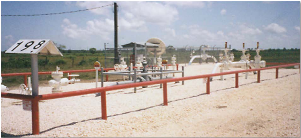
Figure 58: Natural gas pipeline meter and regulator station with pig launcher
