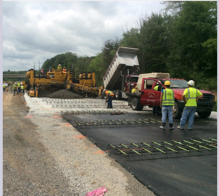
Construction workers apply a Targeted Overlay Pavement solution to a roadway. Photo: PennDOT STIC
