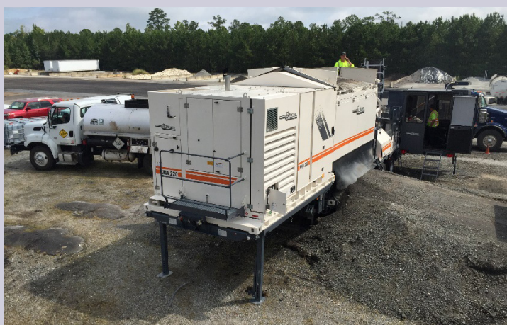
This photo shows CCPR asphalt being mixed in a mobile cold recycling plant. Photo: Mary Robbins
