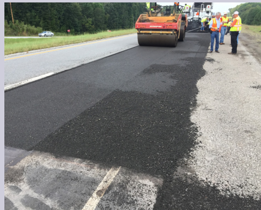
A CCPR mix is being rolled; CCPR is placed and rolled just like traditional asphalt concrete. Photo: Mary Robbins
