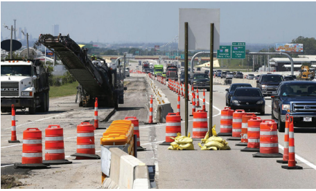
Tulsa often leverages money from the Department of Transportation to help fund stormwater improvements to its road infrastructure.
